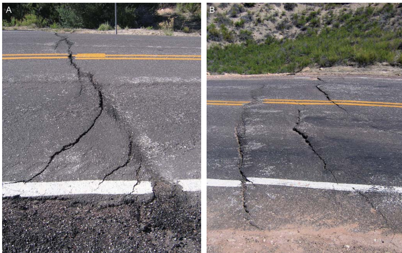
Figure 18. Examples of damage to State Route 9 localized to shear zones that bound landslide 1. A) Left-stepping (diagonal cracks) merging into a nearly continuous right-lateral shear fracture along the west-flank shear zone. B) View upslope of parallel road cracks along the east-flank shear zone. Vertical offset accompanies left-lateral movement. Both photographs taken in May 2007.
