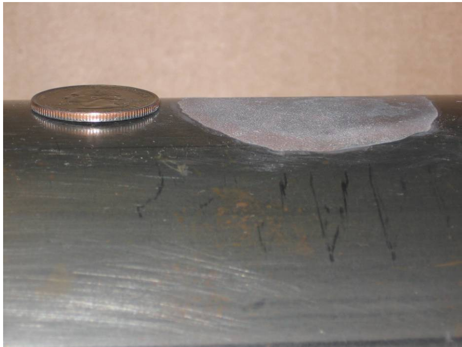
Figure 5.13: Side view of accelerated corrosion, 10% through thickness
