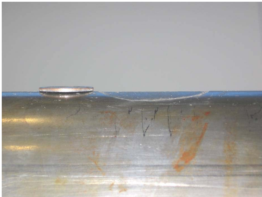
Figure 5.15: Side view of accelerated corrosion, 20% through thickness
