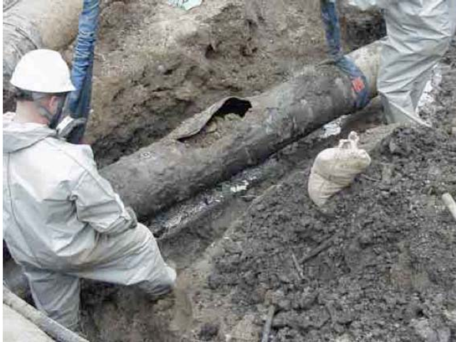
Figure 1.2: Actual rupture in the pipeline (NTSB, 2002)
