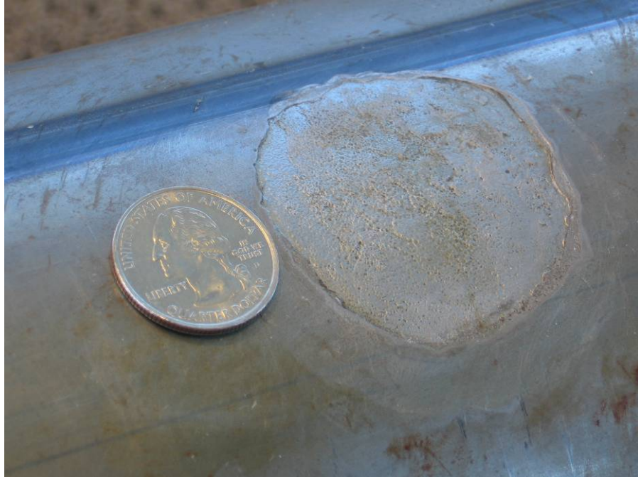
Figure 5.14: Top view of accelerated corrosion, 20% through thickness
