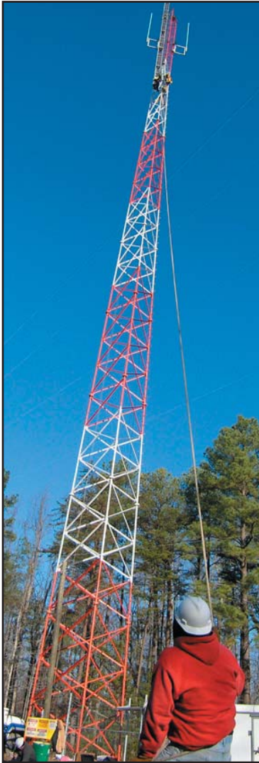
The post Land Mobile Radio tower was constructed in January. Testing for this new radio system begins this month. (Photo by Mary A. Bodine.)
