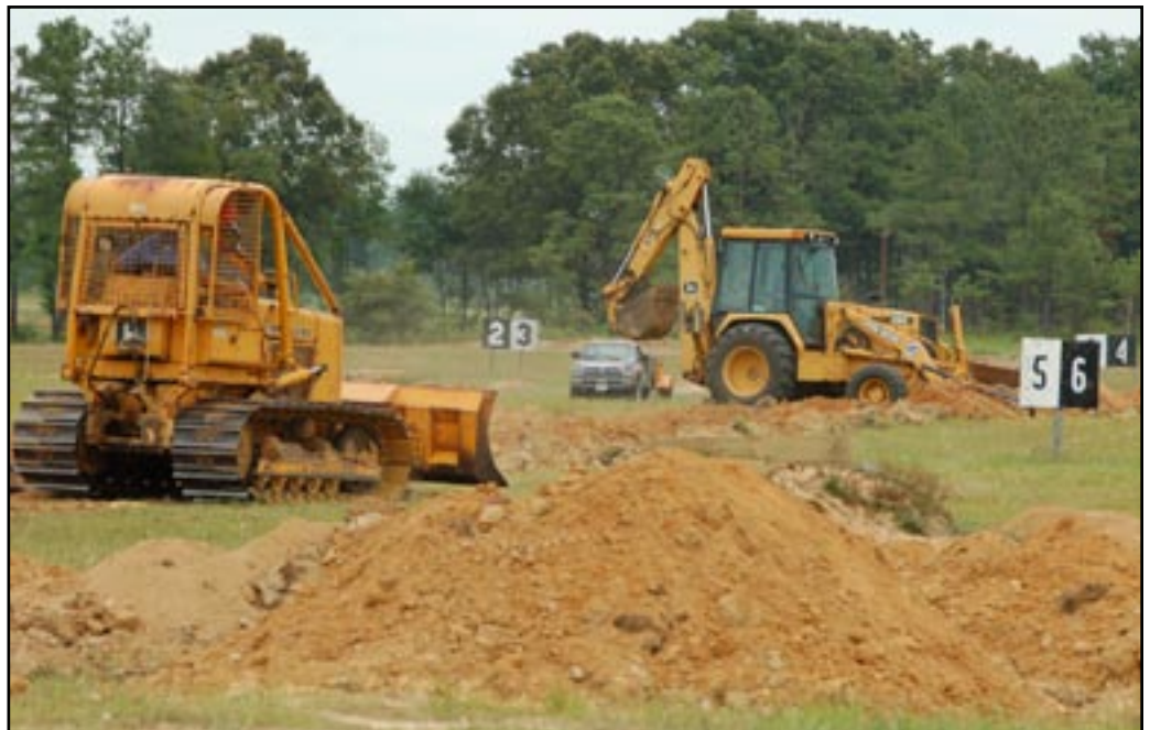
Fort A.P. Hill team members from Range Control and the Directorate of Public Works are currently upgrading Range 32. (Photo by Jason B. Cutshaw)
