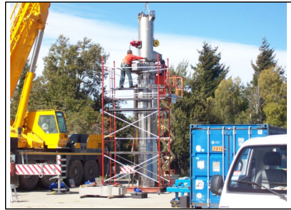
Figure 4: Mounting of DTS on to the LWT at the RA-6 outdoors operation area
