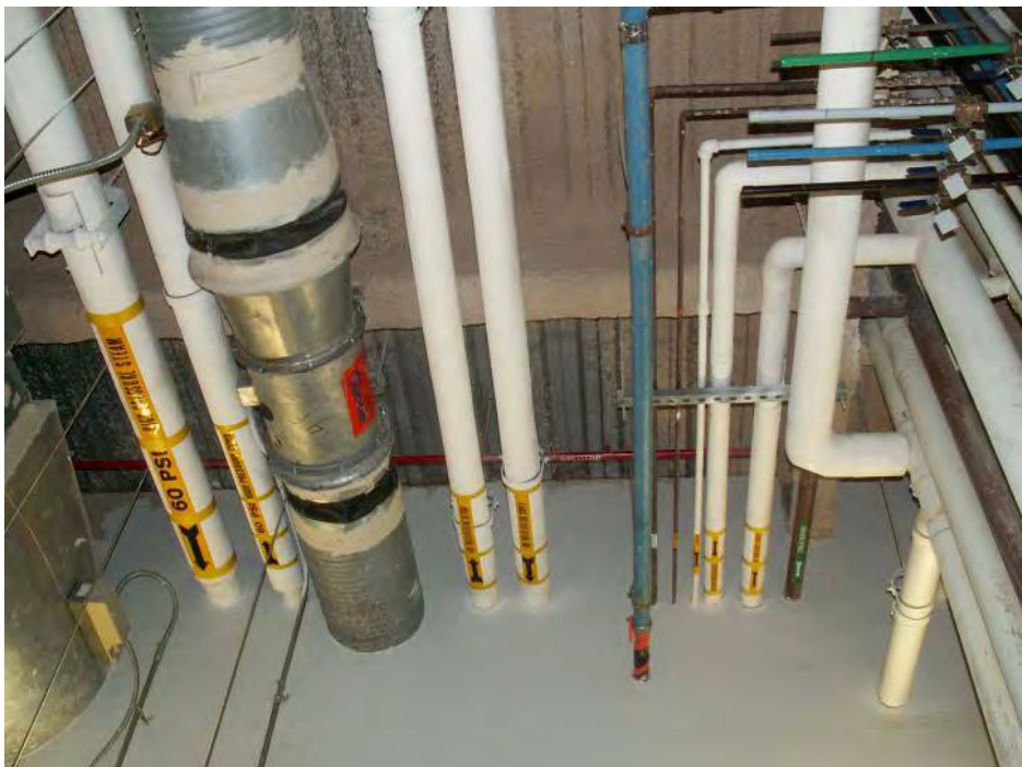
Photo A-4 Service Bay
