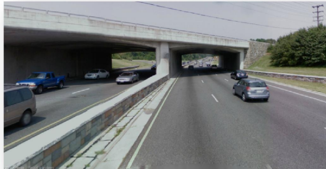
MD 193 Bridge Would Require Reconstruction
