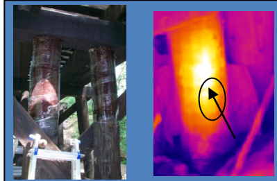
Wrapped pile (left) and infrared image (right)
