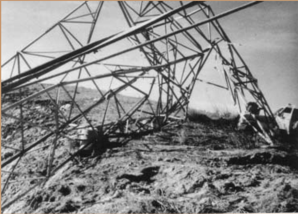
Collapsed Transmission Tower from the 1994 Northridge Earthquake in California
