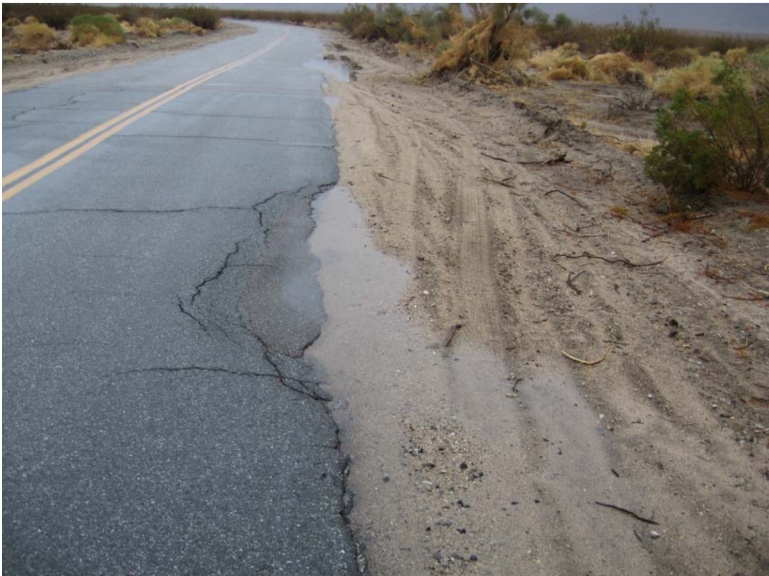
Edge erosion at mile point 13.1
