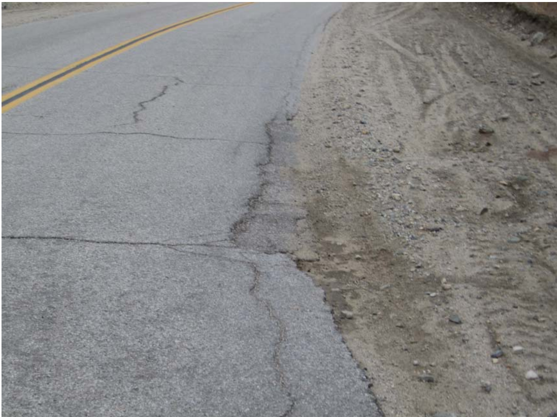
Loss of edge support and edge raveling located near core 6
