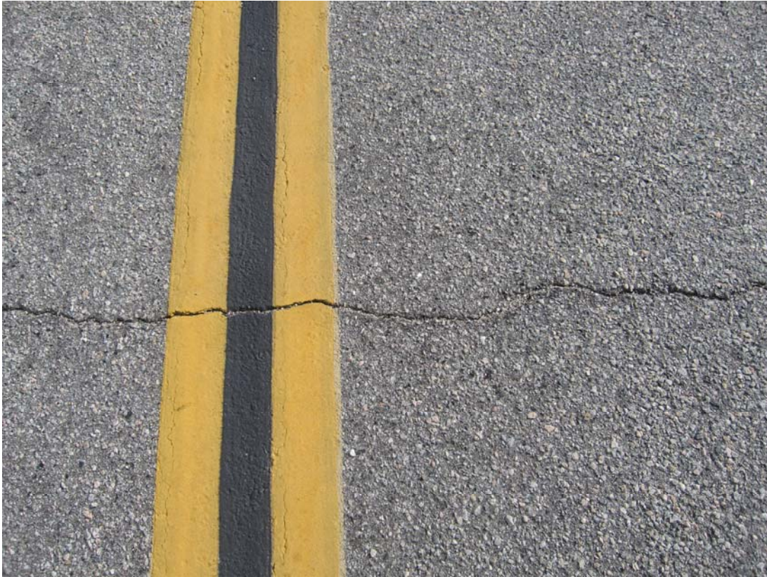
Low severity transverse cracking Located near core 3
