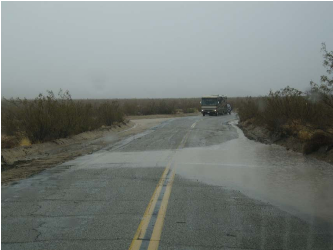
Water Crossing and ponding at mile post 23.2
