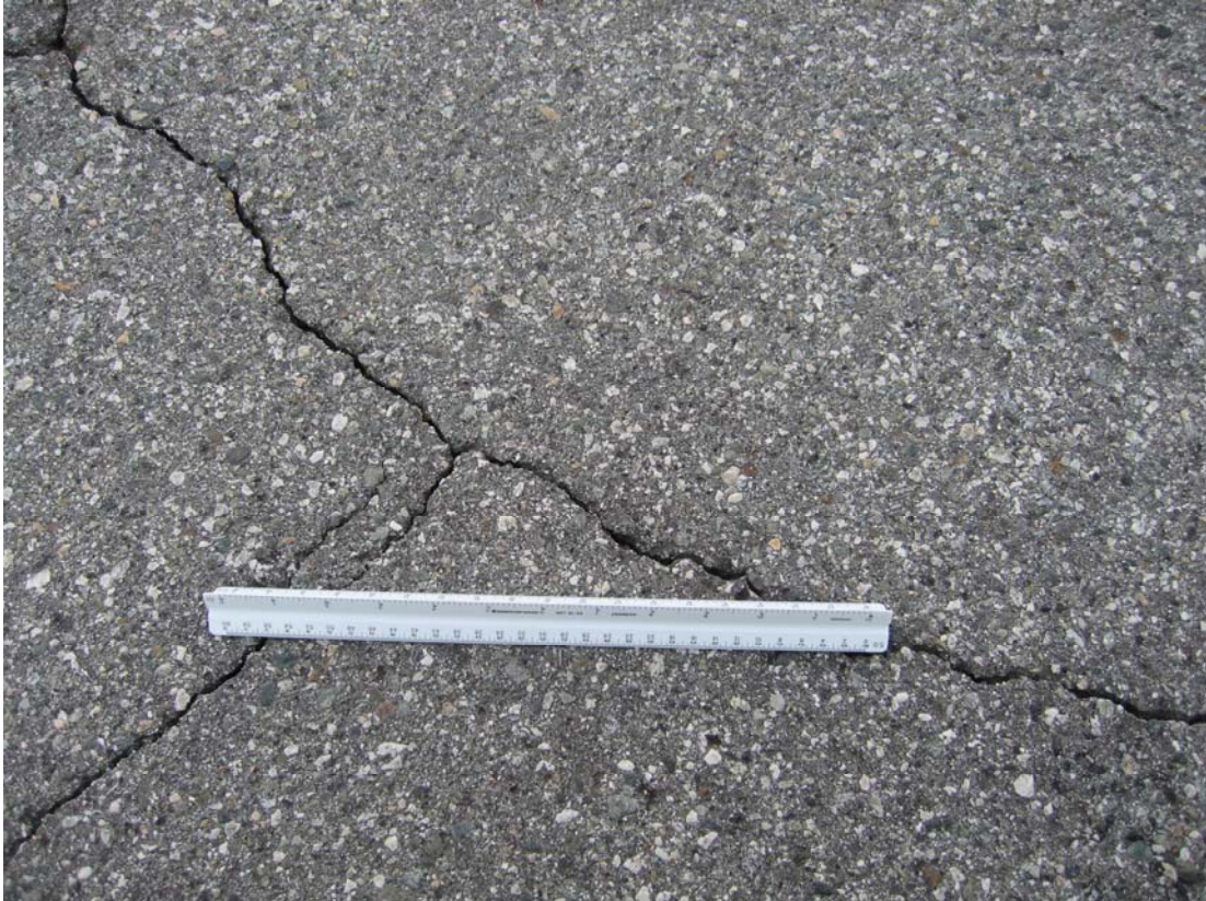
Cracking at core 15
