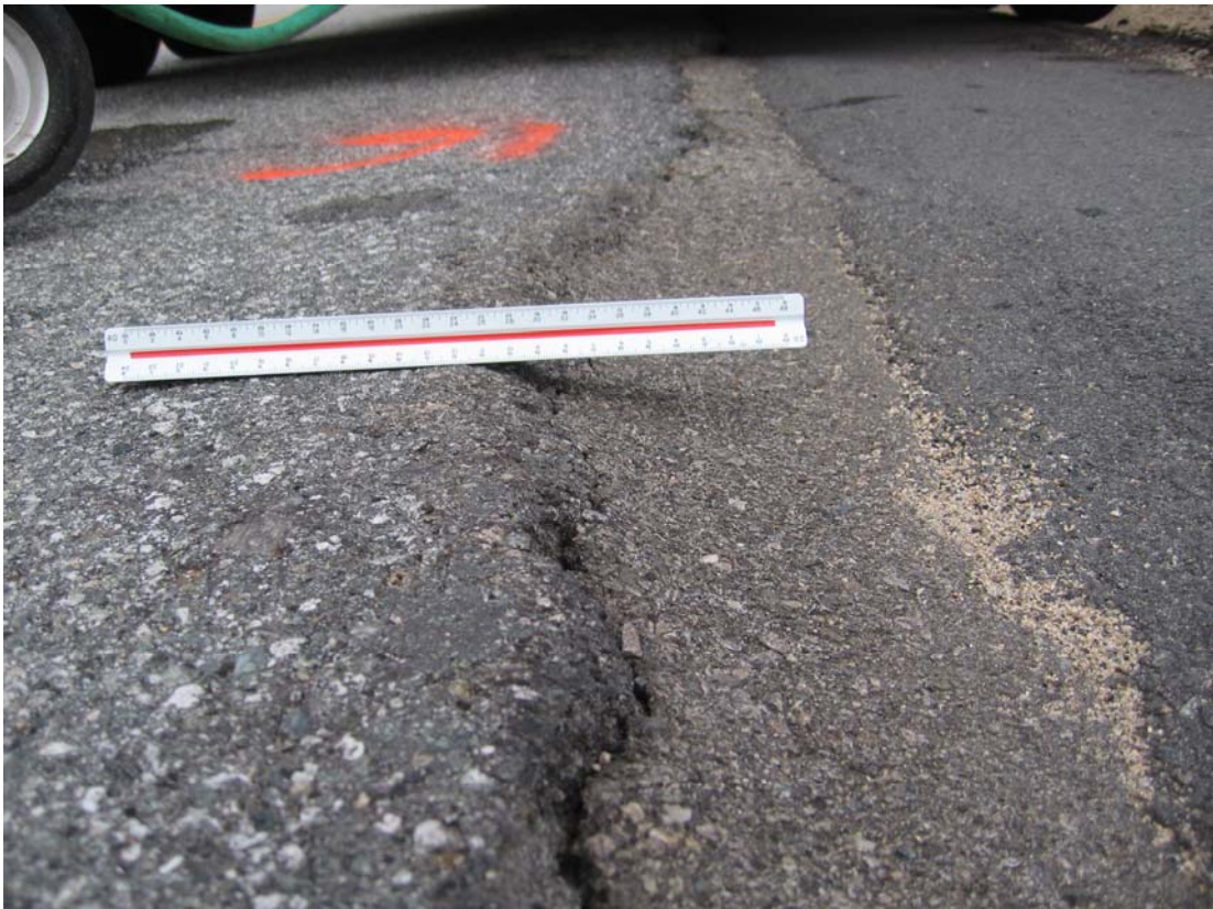
Drop off at edge of pavement and edge repair near core 16
