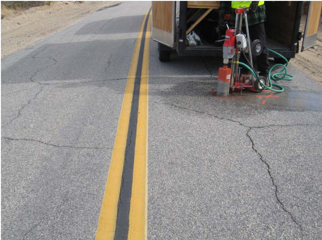
Typical block cracking Located near core 7
