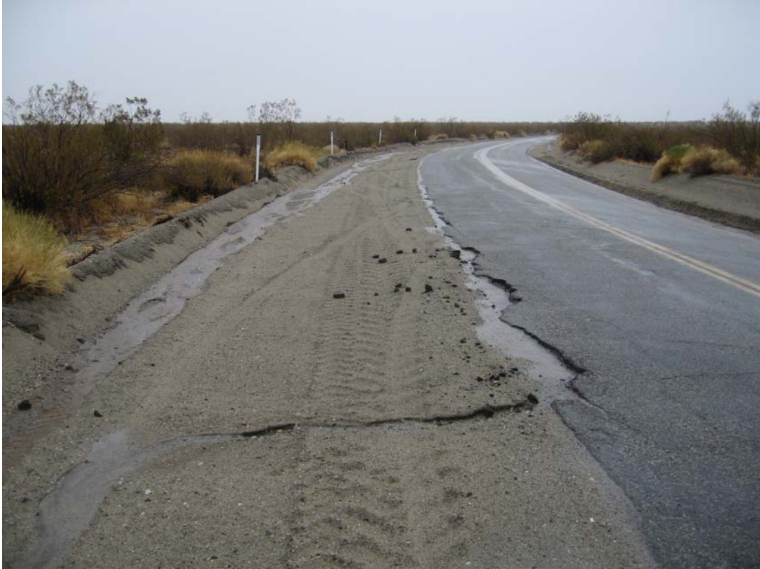
Edge erosion at mile point 19.2
