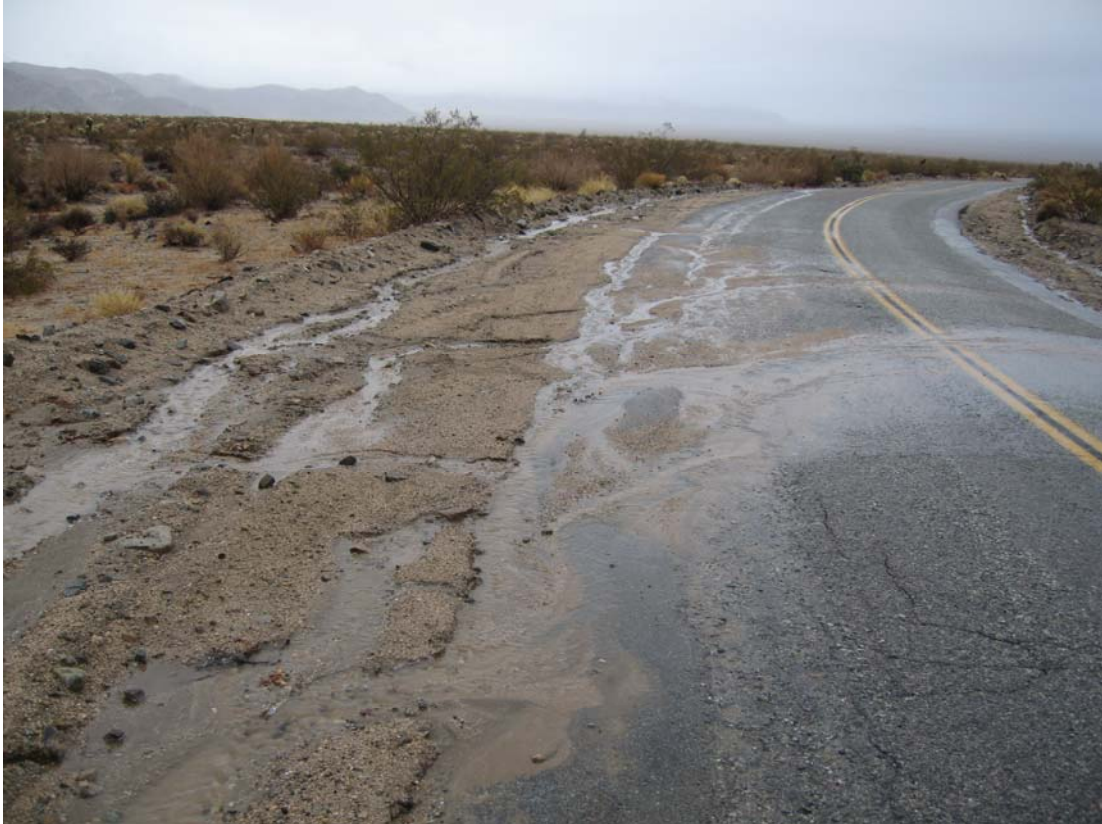
Water Crossing and edge erosion at mile point 10.4
