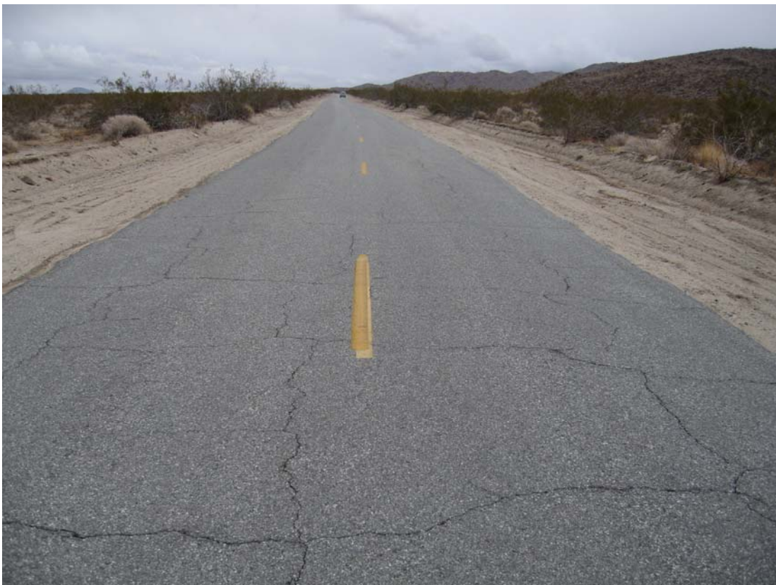
Typical block cracking Located near core 8
