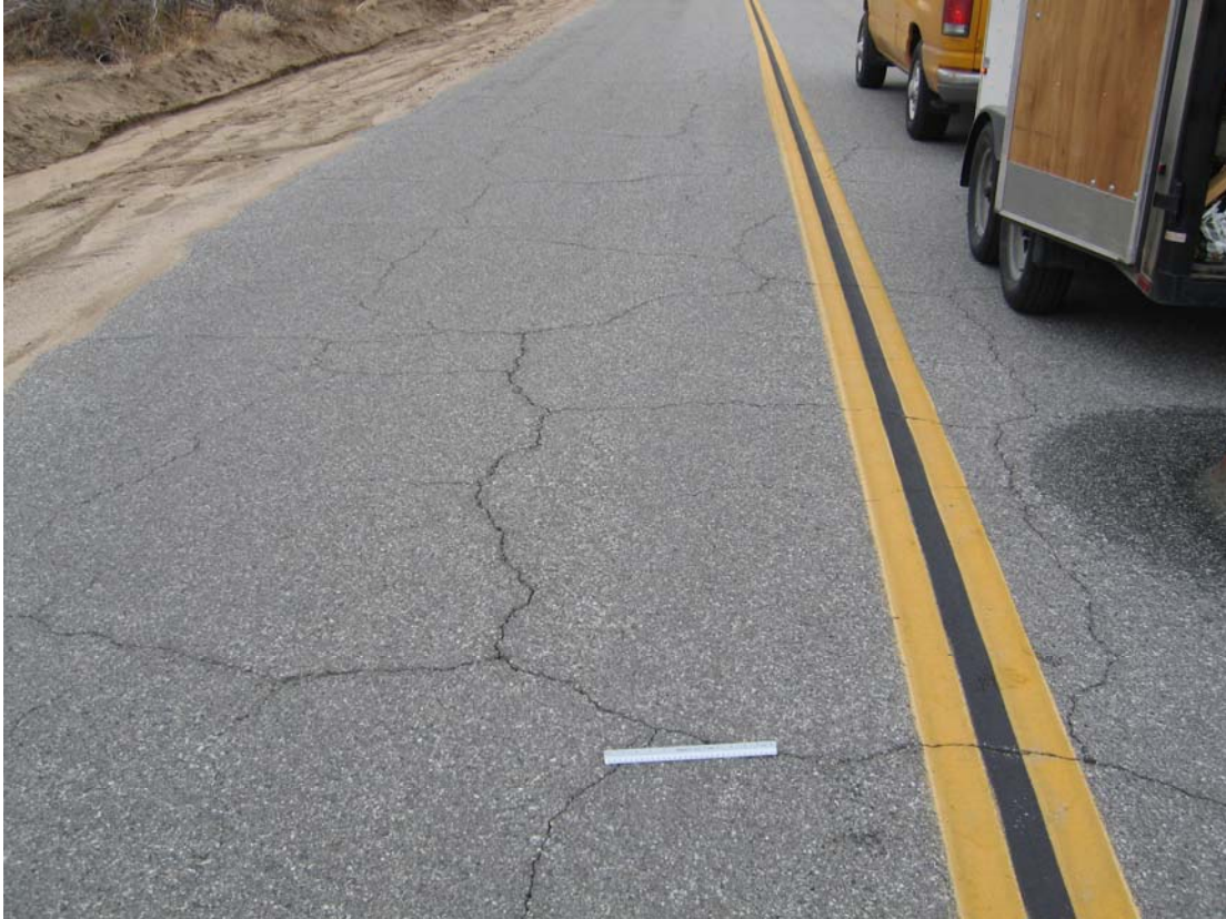
Block cracking at core 15
