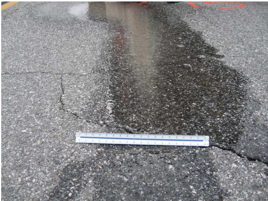
Low severity rutting at core 15
