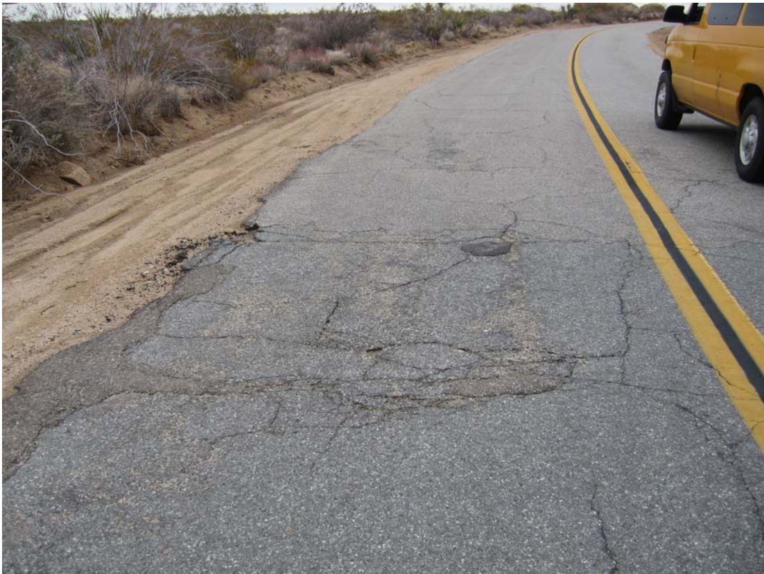
Block cracking, fatigue cracking and edge failure at core 17
