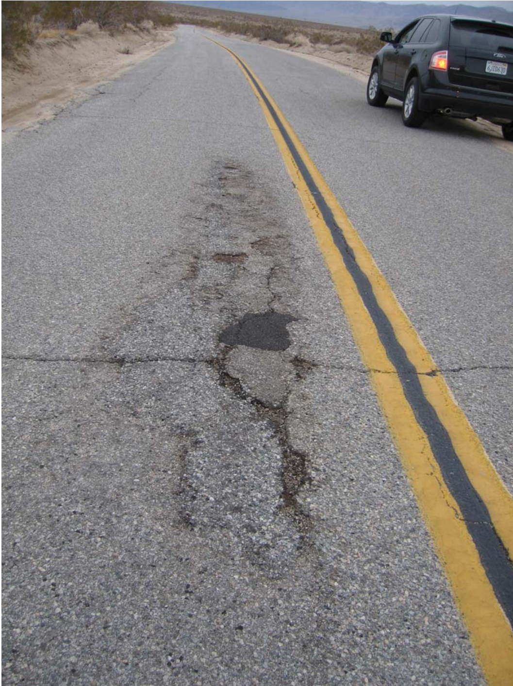
Near core 13 patch distresses
