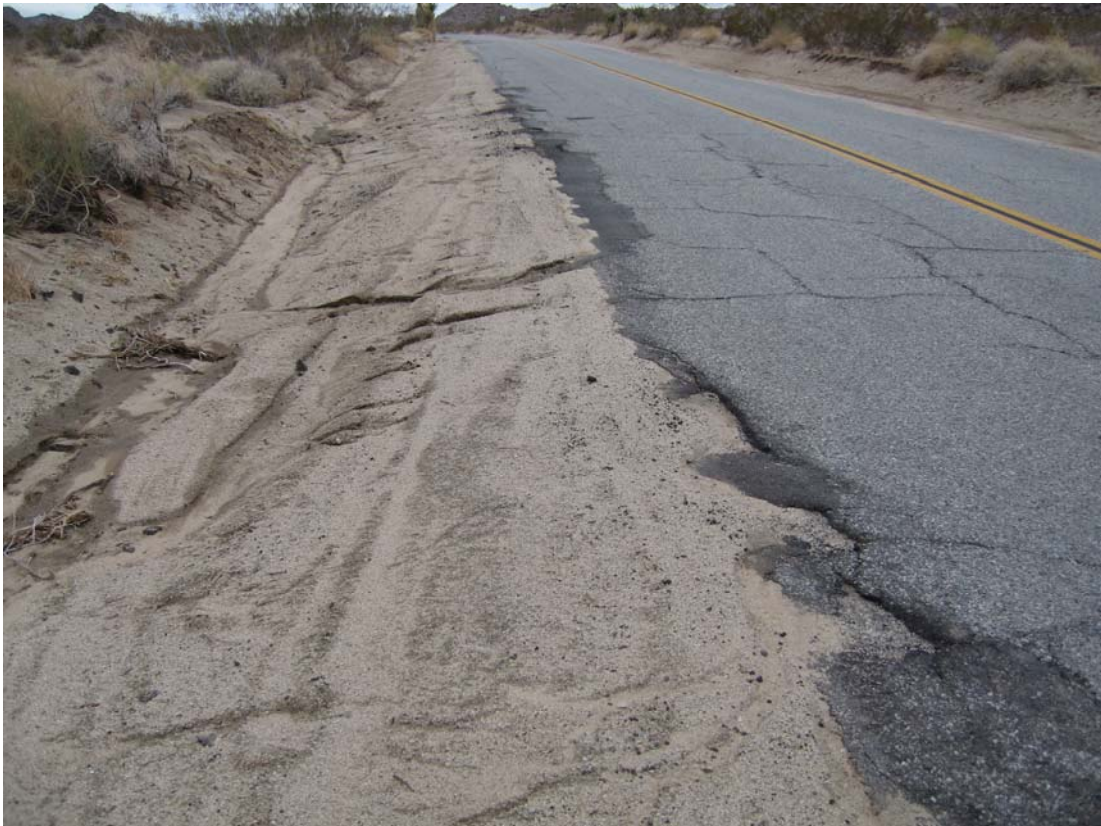
Loss of edge support near Core 13
