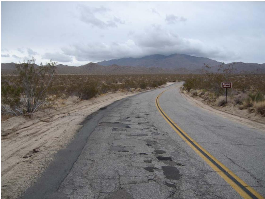
Alligator cracking, patch repair and edge repair near core 14
