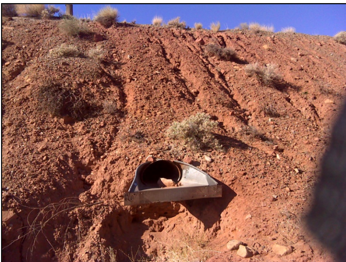
Typical culvert outlet where a gabion drop and revet mattress are recommended for erosion protection
