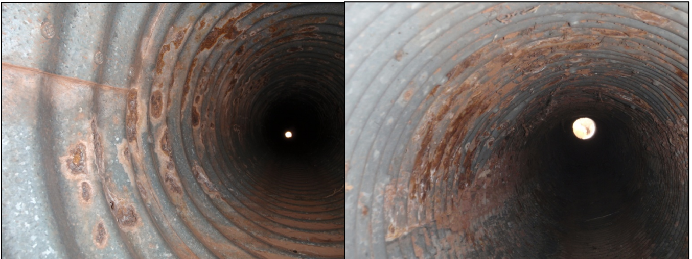
Typical corrosion observed in the 18" CMPs near the campground (Sta 331+24 through Sta 340+60)
