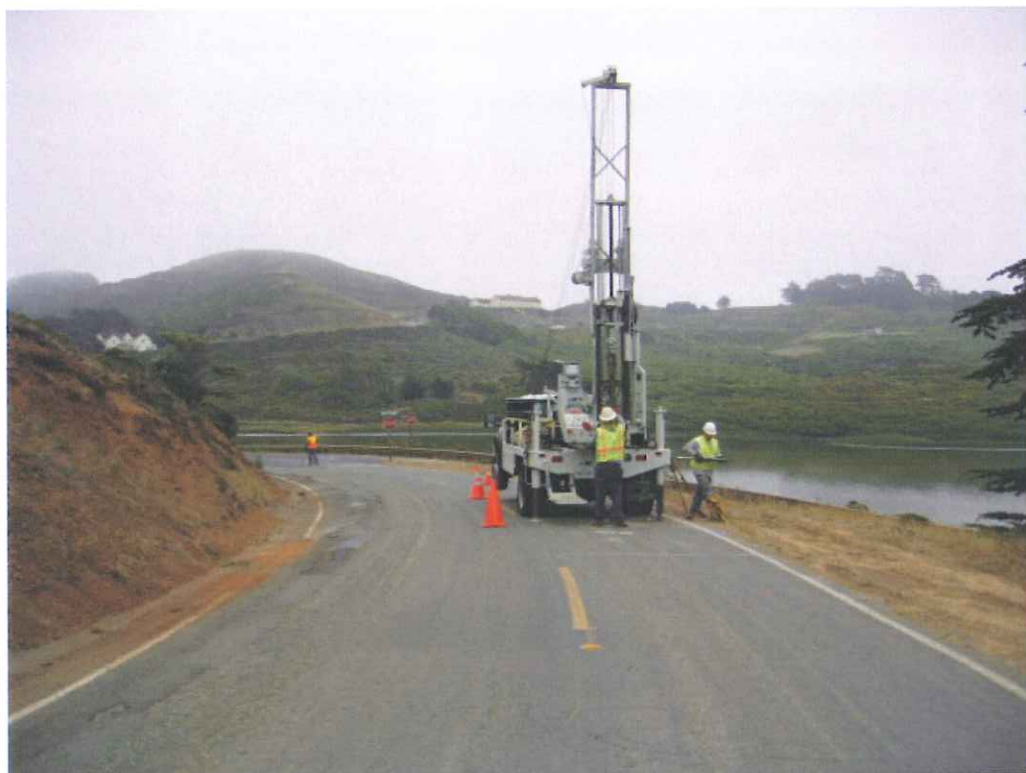
MP 0.25 Old Bunker Road, B-44 near Intersection with Mitchell & Bunker Roads, looking south
