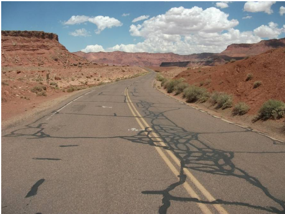
Photo 2 - Start of subgrade problem area near Station 131+00 extra ABC and edge drain recommended
