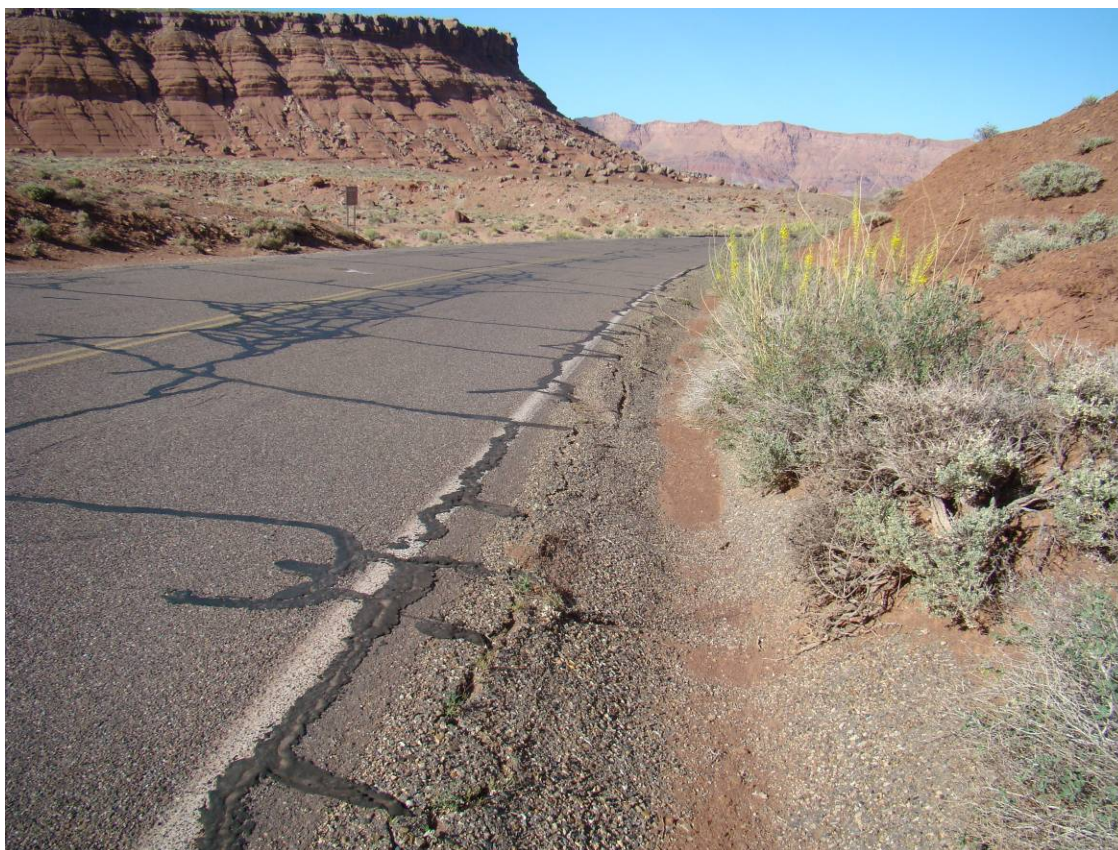
Figure 3.2: Deteriorated ditch pavement, (approx Station 170 - 180)
