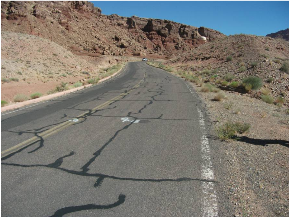
Photo 7 - Near Boring P-18 showing thermal cracks deteriorating to block and utility patch outbound as road descends to Paria River Bridge
