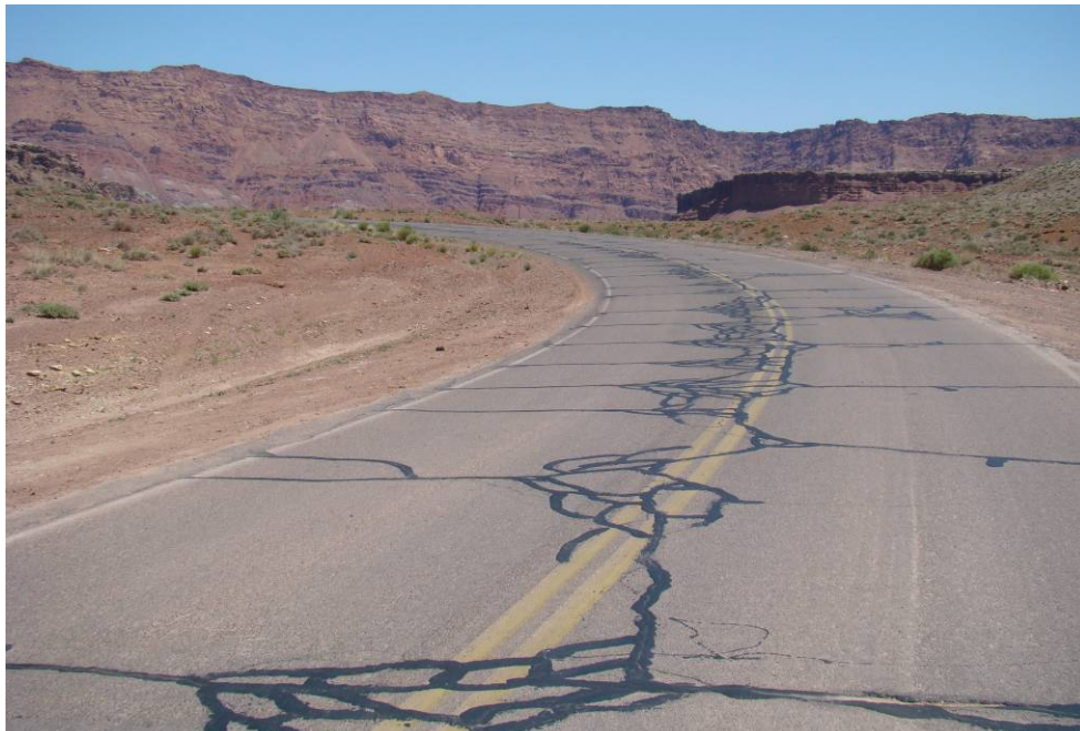
Figure 3.1: Thermal and block cracking patterns at a curve.
