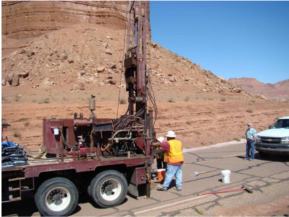
Photo 3 - Drilling P-4 extensive thermal transverse and block cracking in existing pavement
