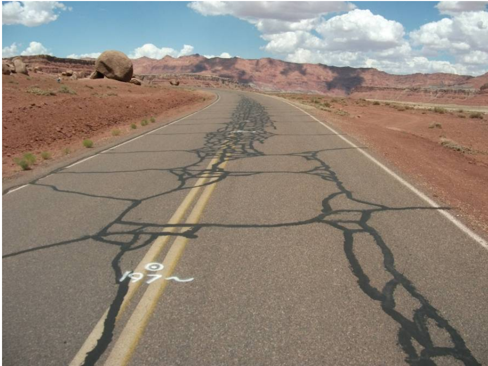
Photo 5 - Typical condition near center of project, thermal cracking with deteriorated center line and some wheel path fatigue cracking
