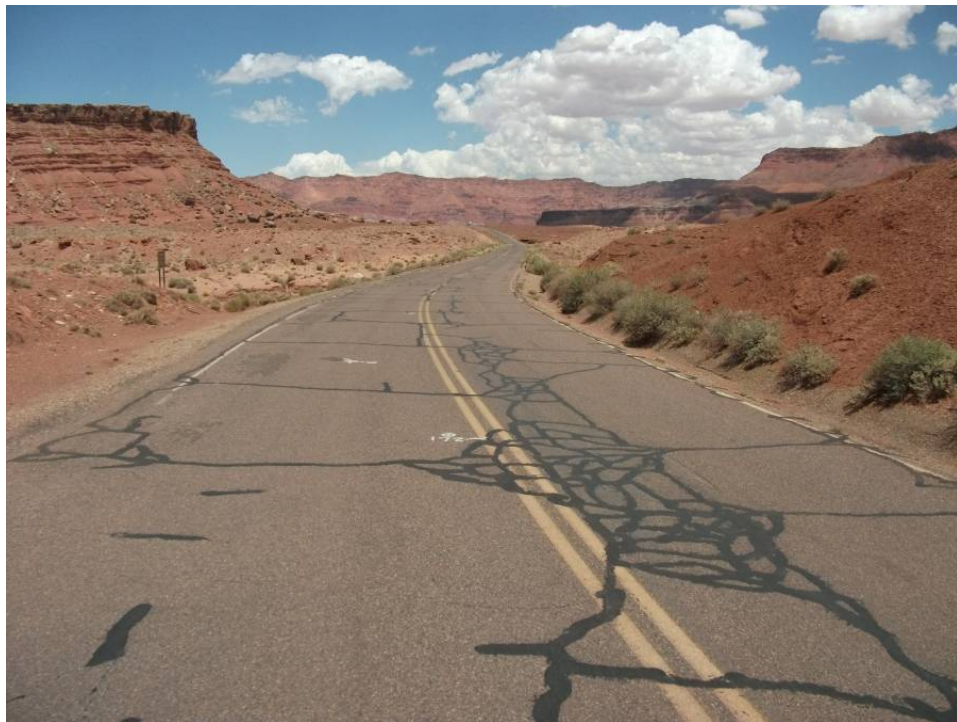
Photo 4 - Lower end of rough section near Sta. 178+00 where edge drain is recommended
