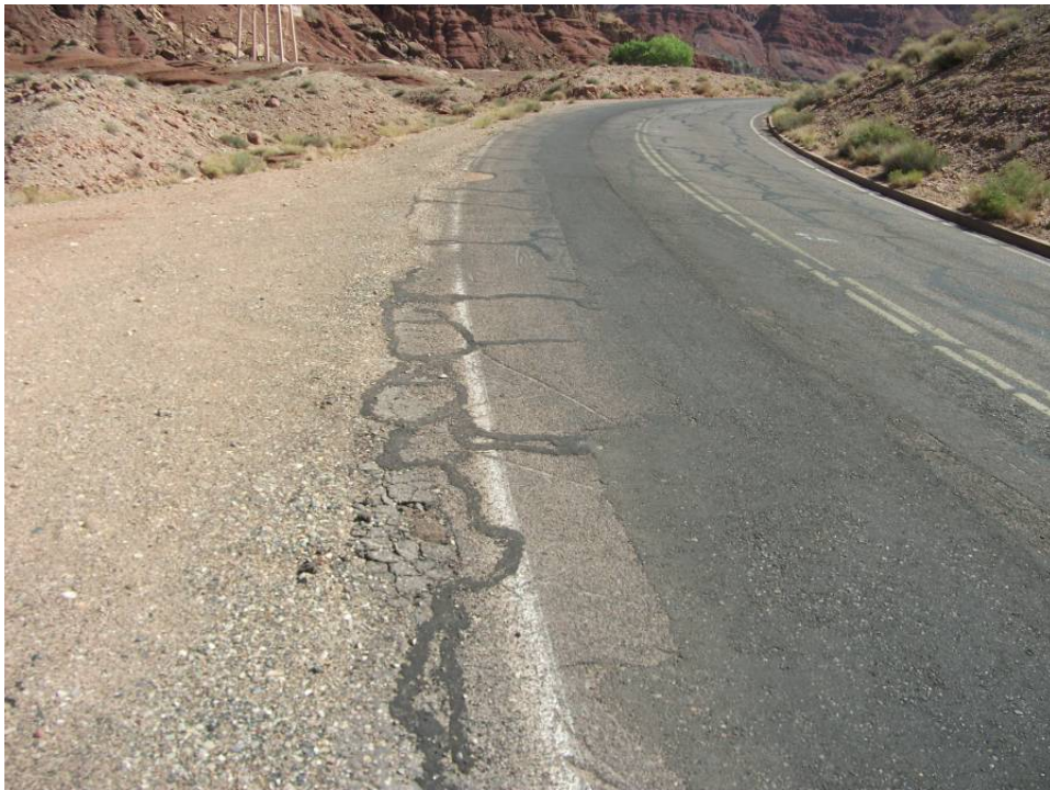
Photo 8 - Edge deterioration and patching from utility installation - block cracking in NB lane
