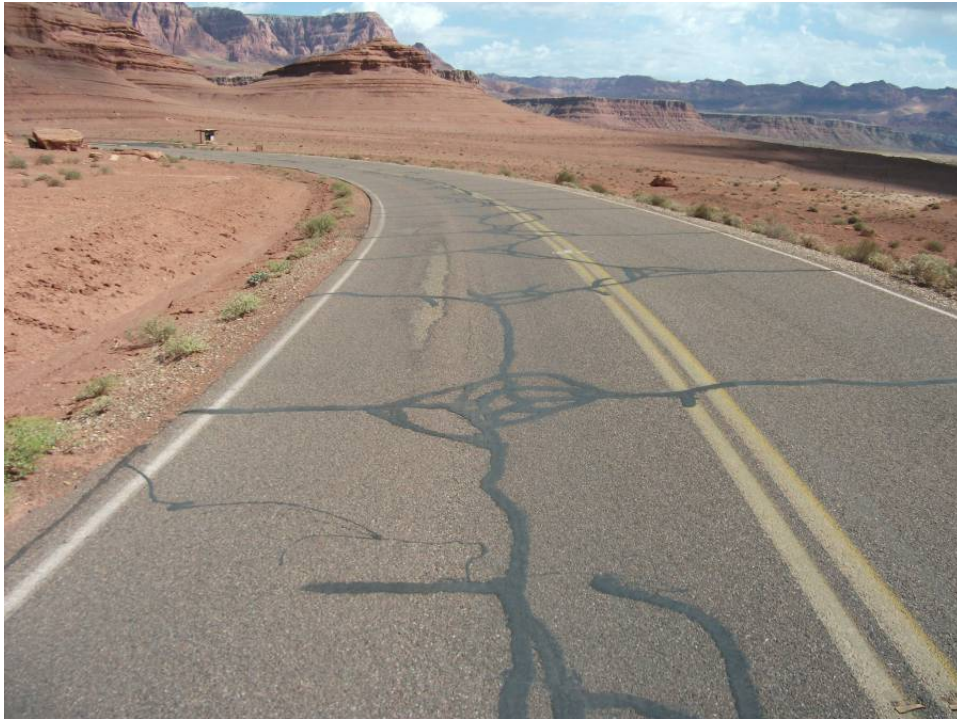
Photo 1 - Typical pavement condition between intersection with US 89 to Pay Station
