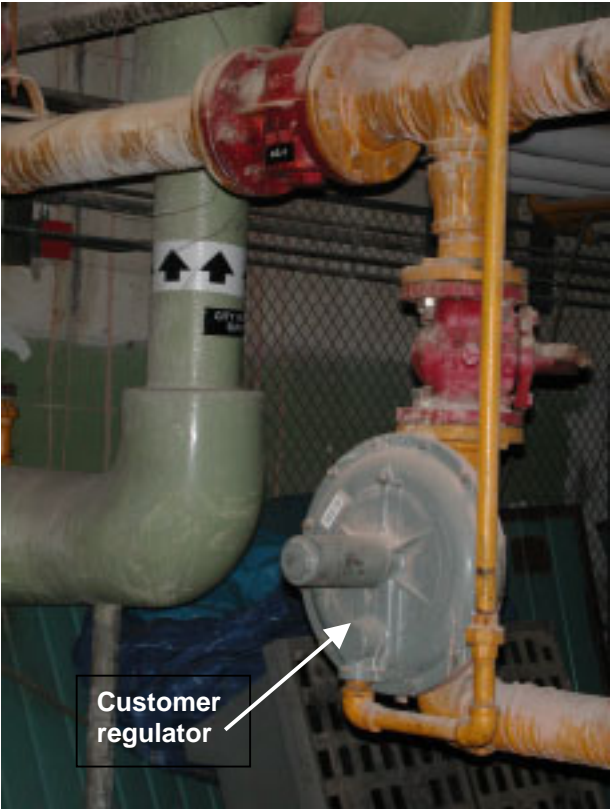
Regulator on the 4-in. Fuel Line Feeding the Furnaces
