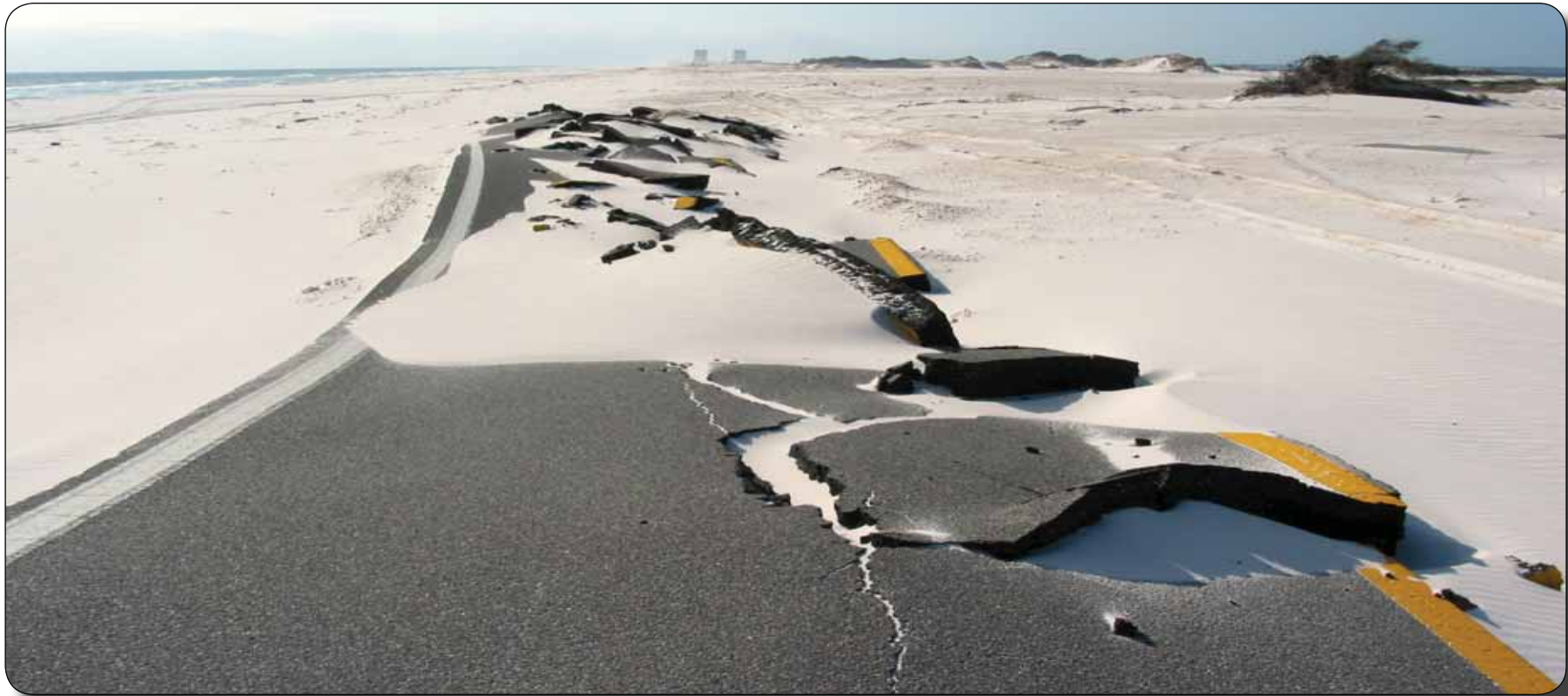
Hurricane Storm Damage, Pensacola, FL
