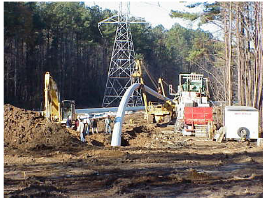
FIGURE 2.2-3 Horizontal Directional Drilling (HDD) Operation (Source: Photo courtesy of U.S. Pipeline, Inc. Reproduced with permission.)
