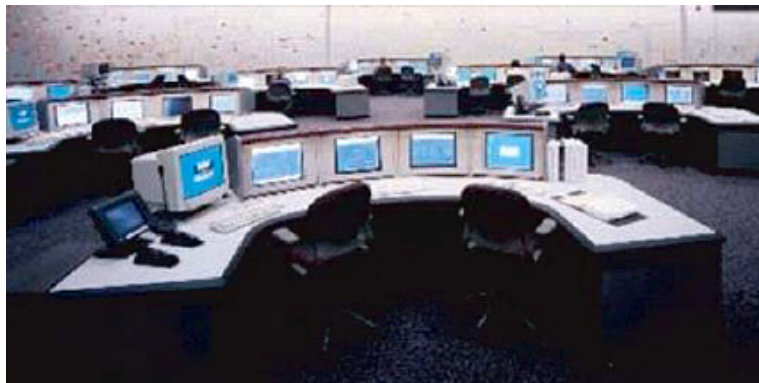
FIGURE 1.2-8 SCADA Center (Source: Argonne Staff)
