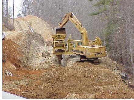
FIGURE 2.1-2 Pipeline Trenching Operations (Source: Photo courtesy of U.S. Pipeline, Inc. Reproduced with permission.)
