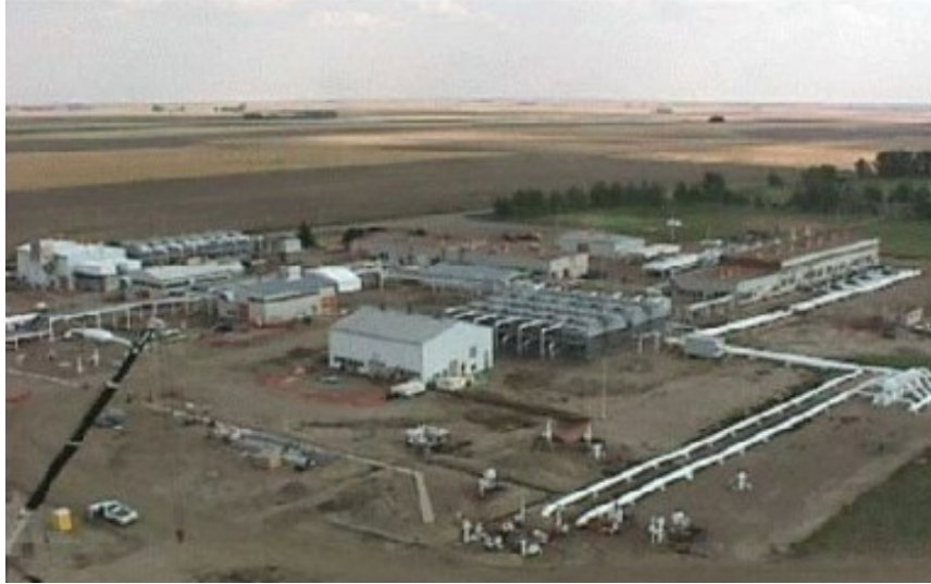
FIGURE 1.2-2 Natural Gas Compressor Station along an Interstate Pipeline (Source: Argonne Staff)
