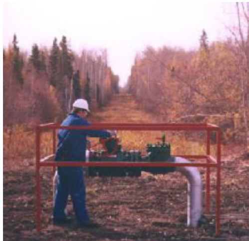
FIGURE 1.2-6 Aboveground Valve on Natural Gas Pipeline (Source: Cirillo et al. 2003)
