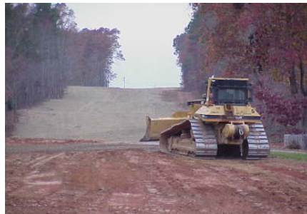
FIGURE 2.1-1 Bulldozer Grading Pipeline ROW (Source: Photo courtesy of U.S. Pipeline, Inc. Reproduced with permission.)
