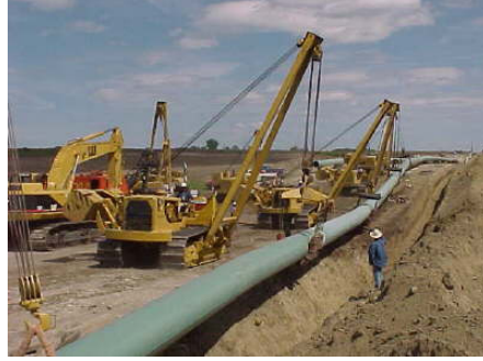
FIGURE 2.1-6 Crew Lowering a Pipeline into a Trench (Source: Photo courtesy of U.S. Pipeline, Inc. Reproduced with permission.)
