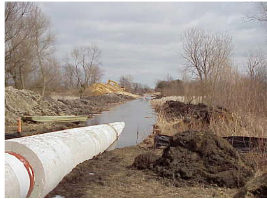
FIGURE 4.1-13 Pipeline for Wetland Installation Encased in Concrete to Counteract Positive Buoyancy (Source: Photo courtesy of U.S. Pipeline, Inc. Reproduced with permission.)
