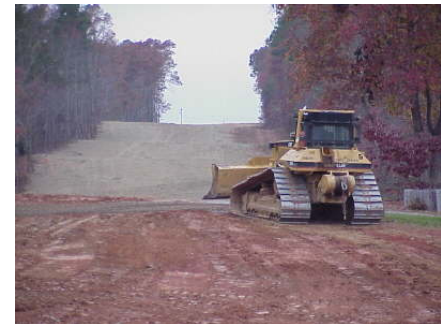
FIGURE 4.1-1 Bulldozer Grading Pipeline ROW (Source: Photo courtesy of U.S. Pipeline, Inc. Reproduced with permission.)
