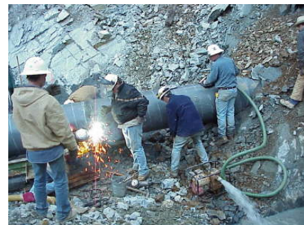
FIGURE 4.1-4 Pipeline Welding (Source: Photo courtesy of U.S. Pipeline, Inc. Reproduced with permission.)
