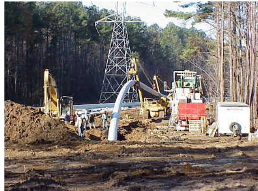
FIGURE 4.1-10 Horizontal Directional Drilling (HDD) Operation (Source: Photo courtesy of U.S. Pipeline, Inc. Reproduced with permission.)
