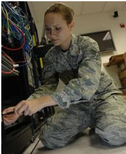
Senior Airman Holly Durkin, a Cyber Surety Technician for the 129th Communications Flight, Moffett Federal Airfield, Calif., replaces an uninterruptable power supply (UPS) from a network server, August 4, 2010. The UPS serves as back-up power supply for network servers in case of main power loss. (Air National Guard photo by Tech. Sgt. Ray Aquino)
