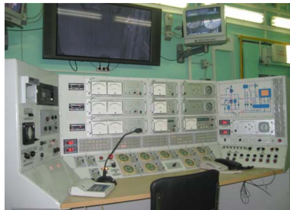
Fig. 3. Control board of the critical facility "Giacint"
