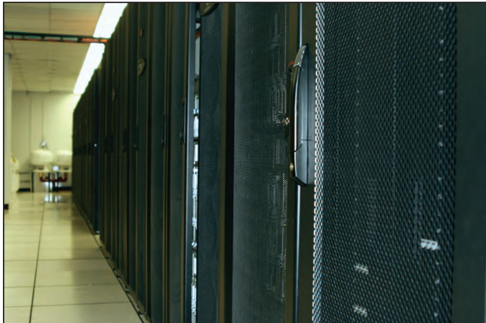
ALTESS' data centers rely on in-row cooling devices and other efficiency measures to reduce power consumption.
