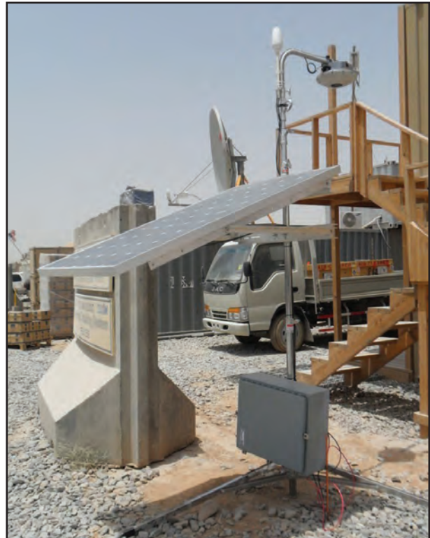
Stand-alone solar-powered (solution for austere locations without commercial power) RFID read capability in support of Surface Deployment and Distribution Command (SDDC) in Afghanistan provides continuous satellite RF-ITV connectivity without sunlight for up to 32 hours.
