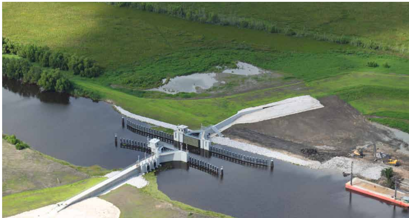
The Western tie-in project along the west bank of the Mississippi River. Photo courtesy of the U.S. Army Corps of Engineers.
