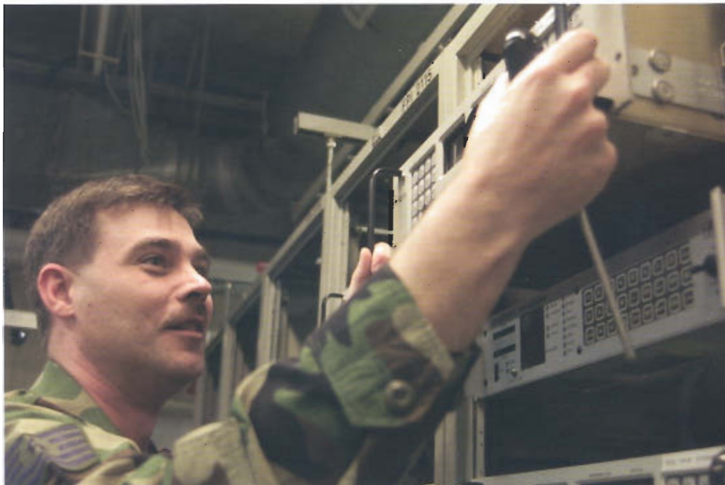
Tech. Sgt. Joseph Brown, 52nd Communications Squadron Operating Location-C Global Weather Spangdahlem Air Base, Germany. Sergeant Brown, 52nd CS OL-C chief, pulls out a high frequency radio receiver from a rack at Pruem Air Station Apr. 23. The GWIP mission at Pruem AS recently ended and the installation is slated to close this summer. Photo by 1st Lt. Gerardo Gonzalez.
