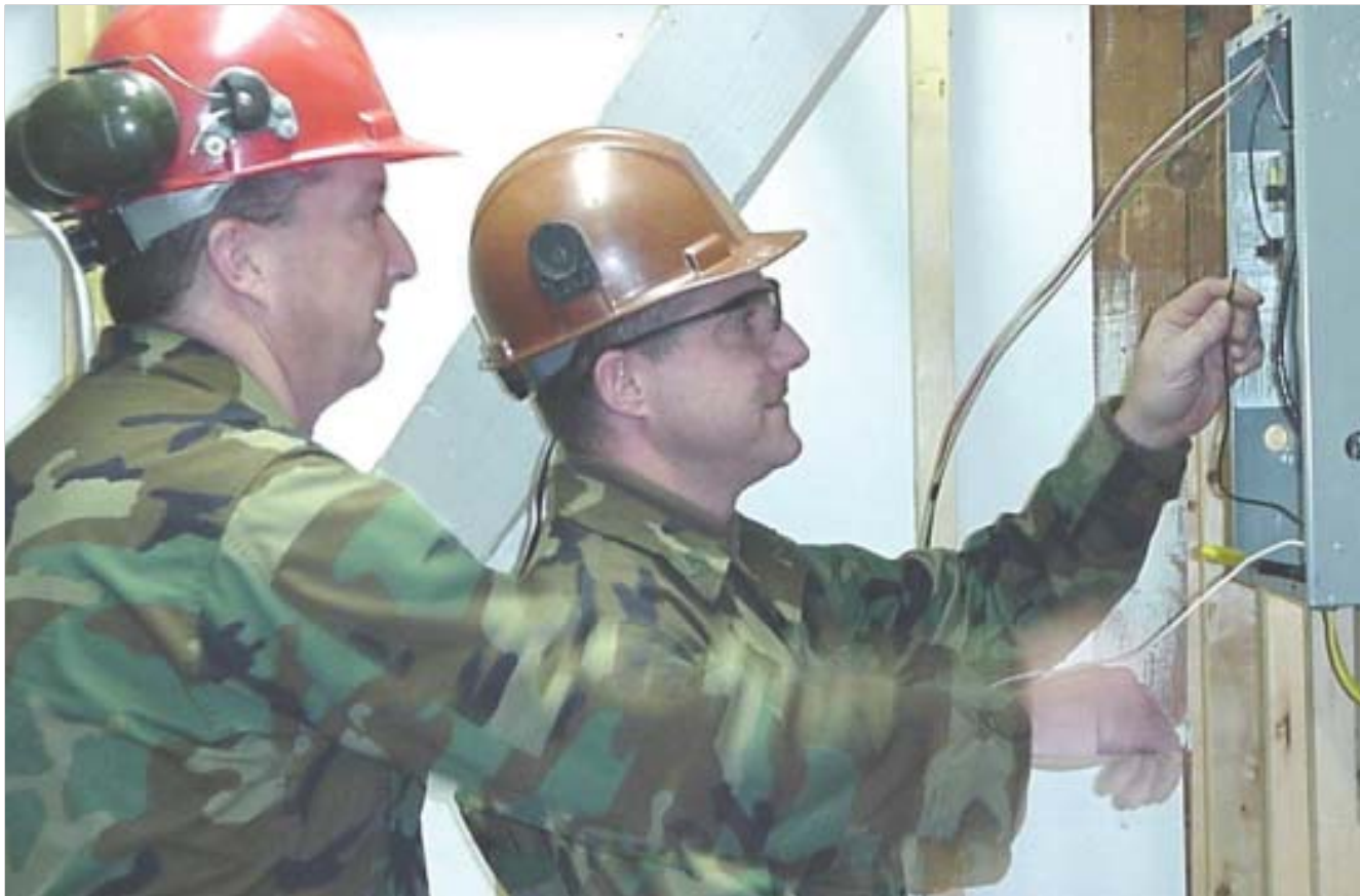
Master Sgt. Kevin Keefe (left) goes over the workings of an electrical panel with a student.
