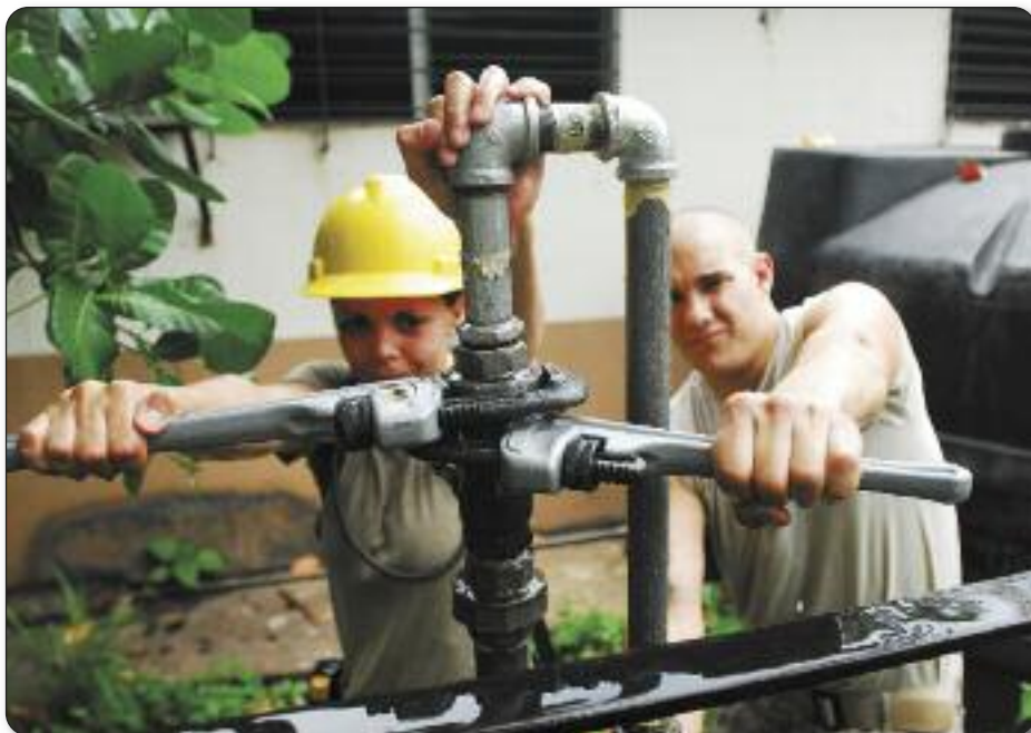
Pfc. Megan Cullen, Penacook, and Pvt. 2 James Lafond, Raymond, of the 160th Engineer Company of Concord, tighten a pipe together as the water pump is tested outside the Tecoluca General Medicine Clinic in San Vicente, El Salvador, on May 23. Photo: Spc. Karin Leach
