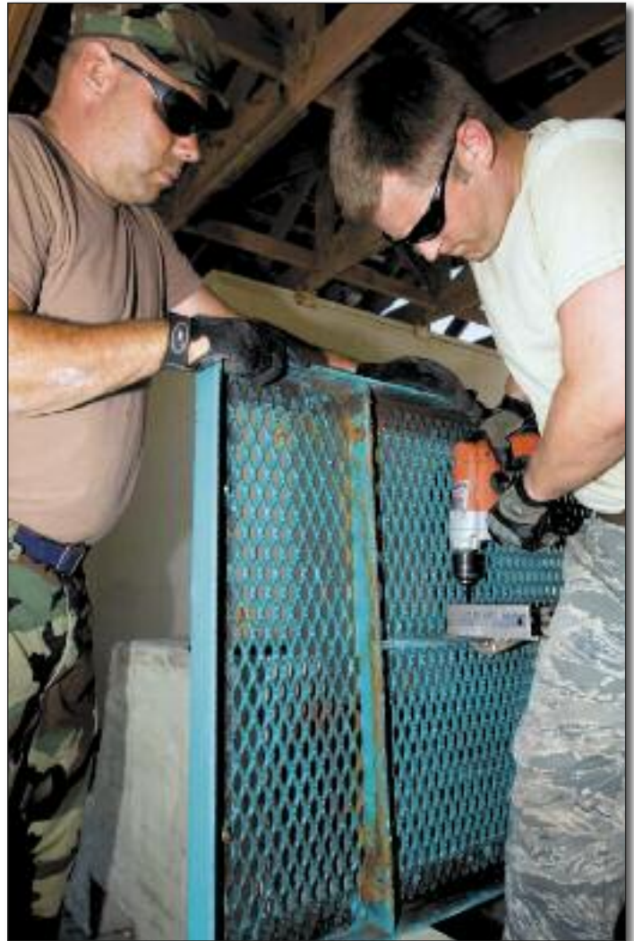
Master Sgt. Todd Buttrick and Airman 1st Class Mark Quinn, members of the 157th Civil Engineering Squadron, secure a metal bracket to a tabletop at Windmill Beach, Aug. 10. The 157th CES is deployed to Joint Task Force Guantanamo for two weeks of training. JTF Guantanamo photo: Army Sgt. Andrew Hillegass
