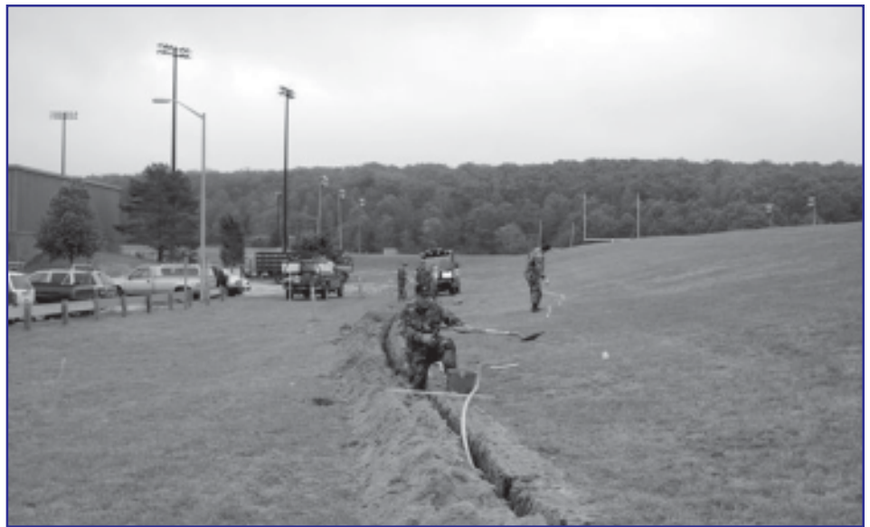
Master Sgt. Guy Chiocchio, who ran the scoreboard installation project, climbs out of the trench after smoothing it to install electrical conduit.
