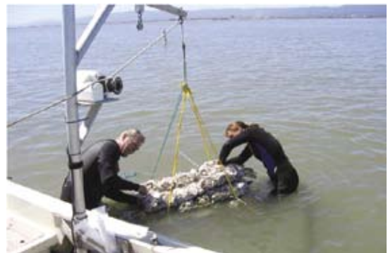
Biologists install bagged Pacific oyster shell reefs at the Marin Rod and Gun Club restoration site in San Rafael.
