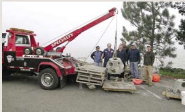
A crane lifts Reef Balls™ for placement into offshore intertidal and subtidal areas.
