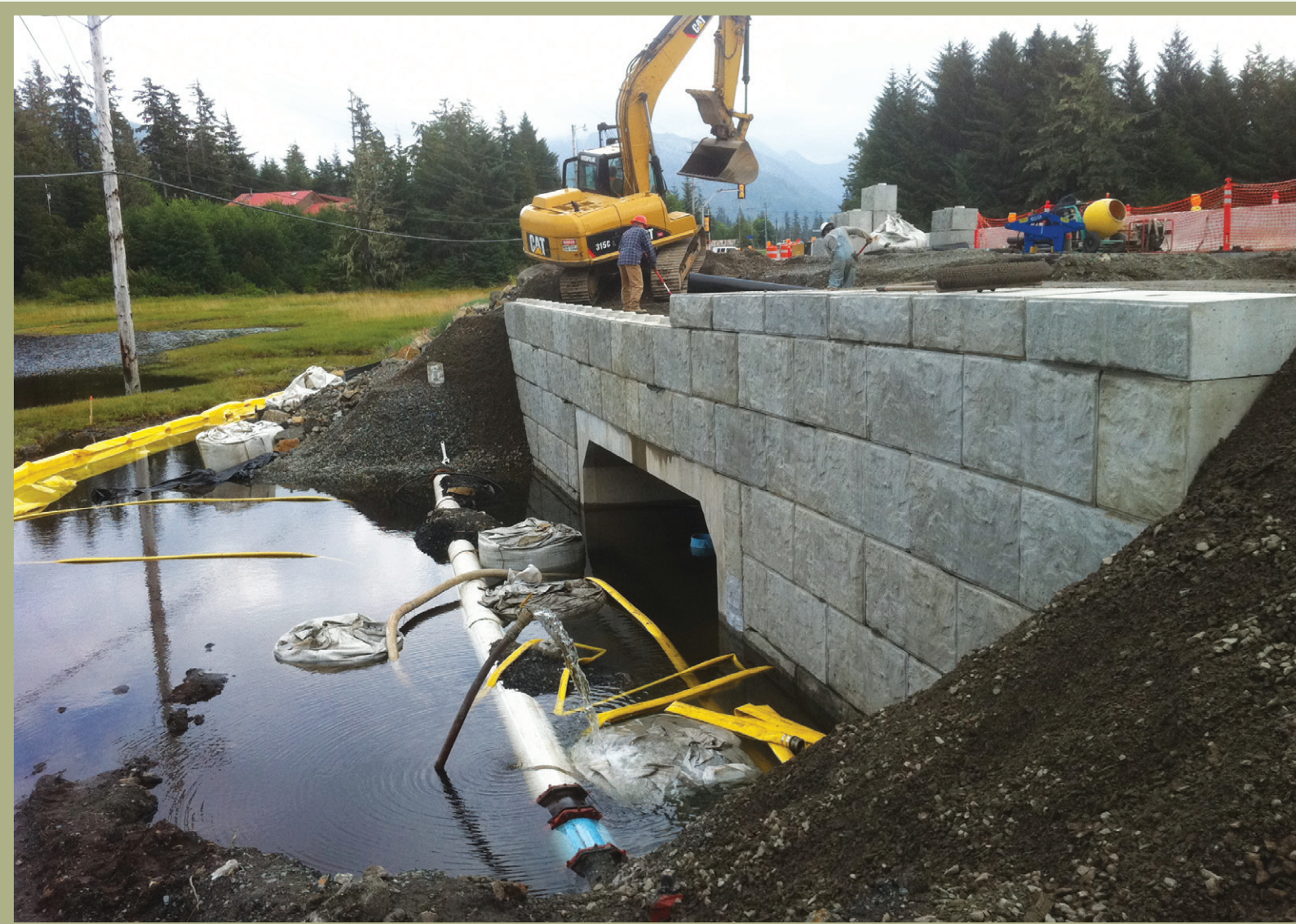
Construction of a larger culvert at the Klawock Highway. © Rob Bosworth, TNC
