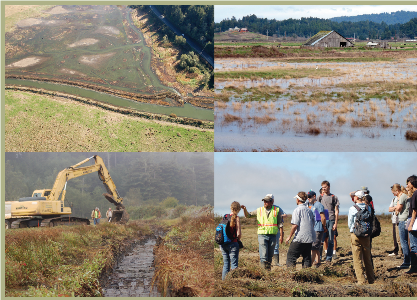
Top left: Post-restoration aerial view of natural tidal inundation into former pastureland, © Lindsay Magnuson. Top right: Tidal inundation providing habitat to juvenile salmon, © Aldaron Laird. Bottom left: Slough channel excavation during project, © Linda Serrano. Bottom right: Applied Ecological Restoration tour to student group, © Rob Holmlund.
