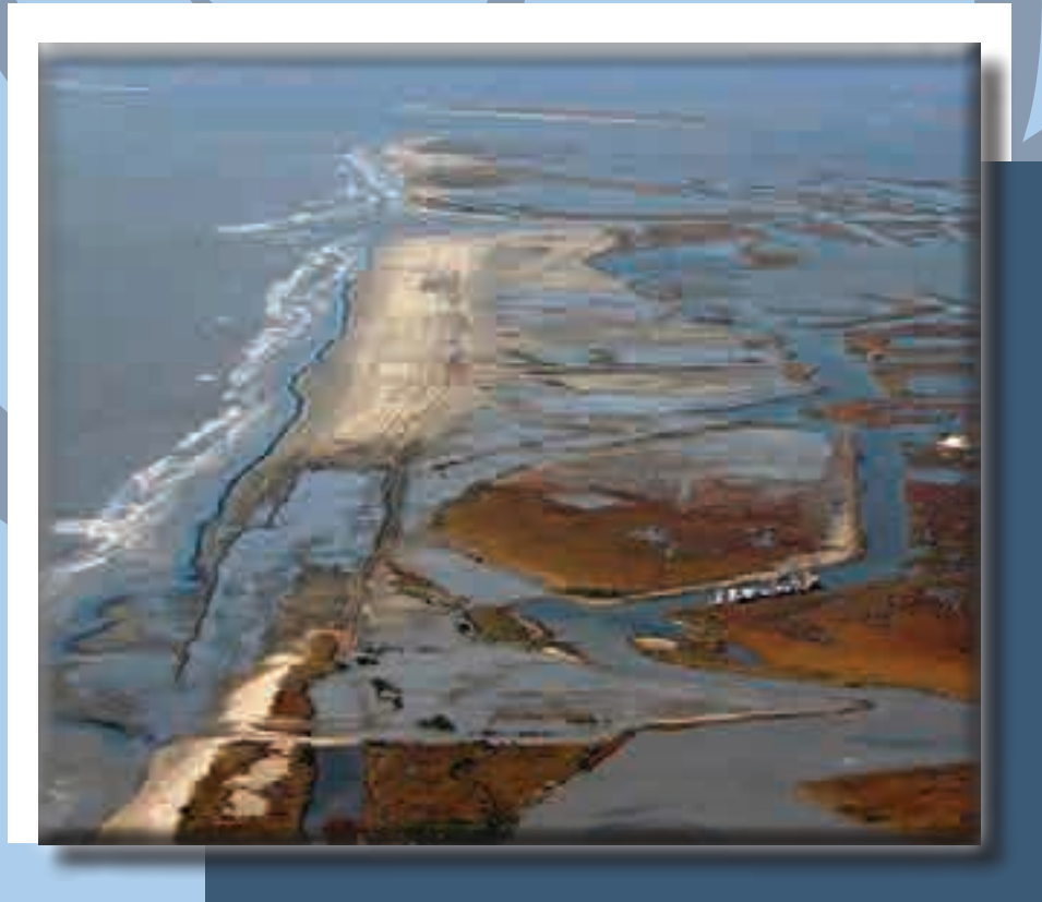
Midway through construction, this island within 2 years matures into a fully functional barrier island (middle right photo).
