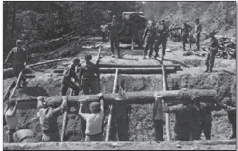
Engineer students building a wooden bridge across a stream at Fort Belvoir, 1963.
