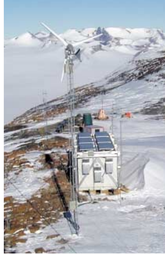
Northern Power Systems/PIX08958
