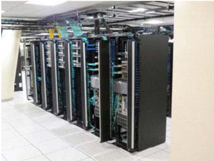
Figure 2. The data center at NCWCP.
