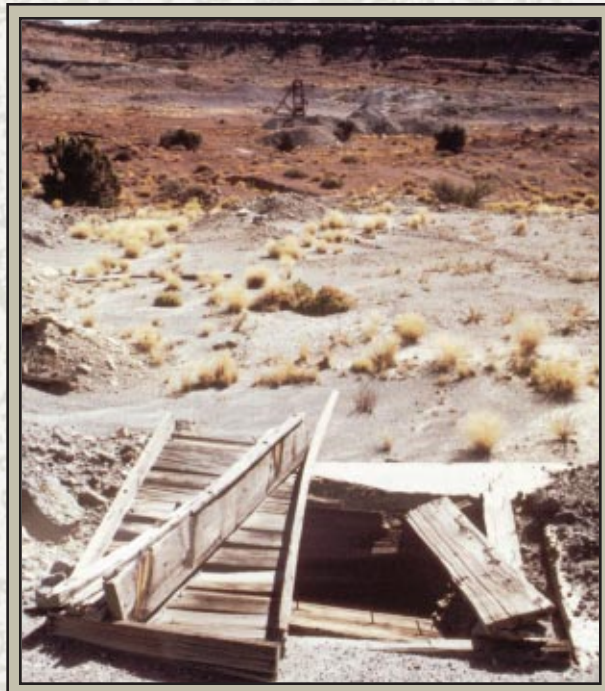
The deteriorated condition of wood at the surface hints at the poor condition of supports within the underground mine.
