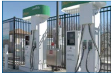
Hydrogen fueling station in Hempstead, Long Island
