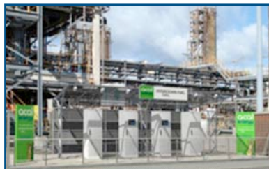
Fuel cells installed at the Solvay plant in Belgium
