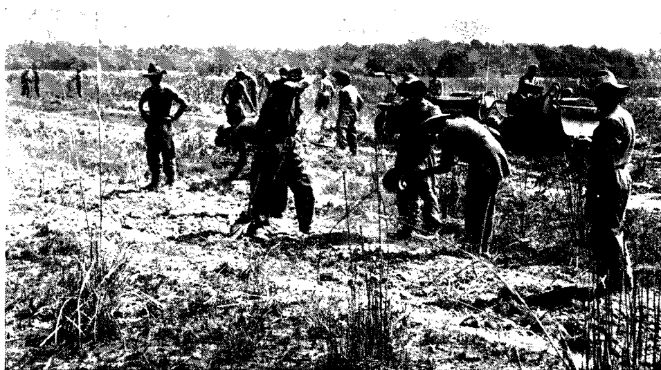
Engineers flown in by Col. Philip G. Cochran's Air Commandos are seen constructing a landing strip behind Japanese lines in Burma for planes of the Troop Carrier Command. The completed airfield was capable of accommodating C-47s and gliders bearing invading troops and equipment.
