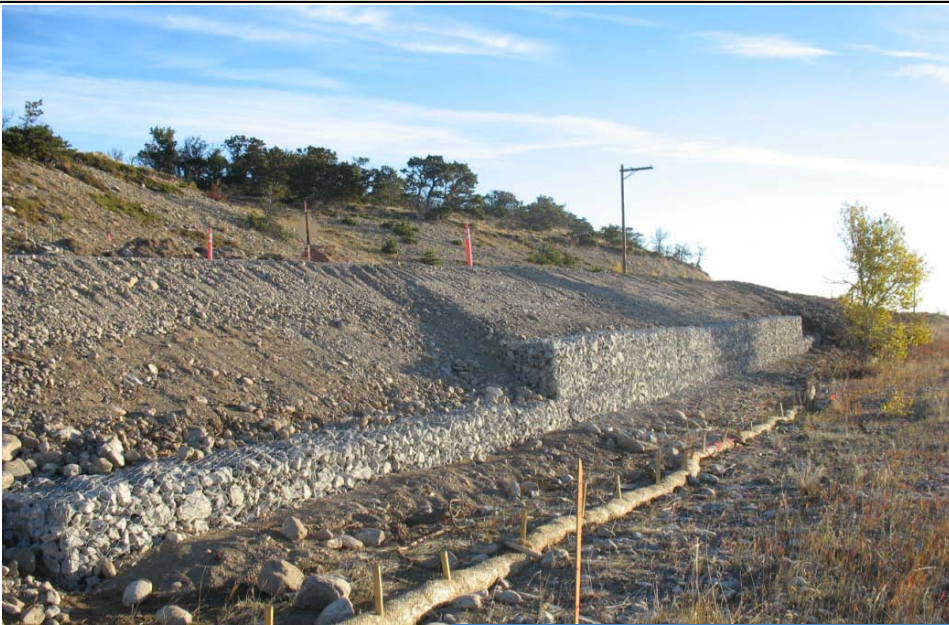
Area of finished gabion wall installation. Slope finishing work still remains in this area.
