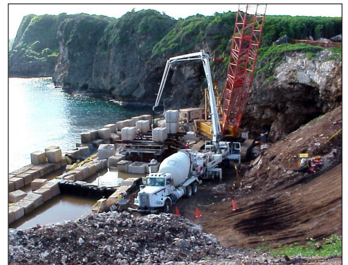
Photo, right: Initial stage of sea wall construction at Orote landfill. (US Navy)
