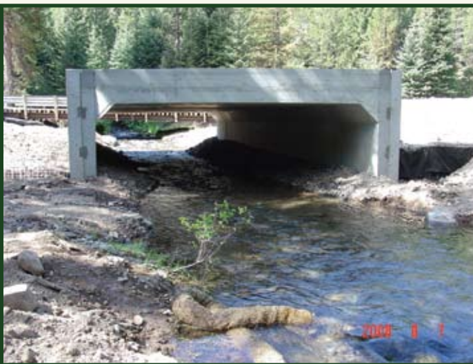
Looking upstream at partially completed structure during Construction – note temporary bypass bridge in background.
