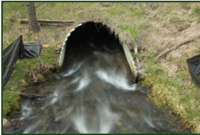
Before: looking downstream at the culvert inlet – note constriction of the stream as it enters the culvert in this 2-sec. time-exposure photo.
