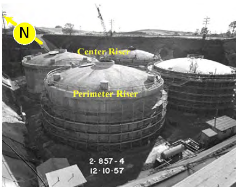
Figure 2.1-2: Dome and Risers on Type IV Waste Tanks
