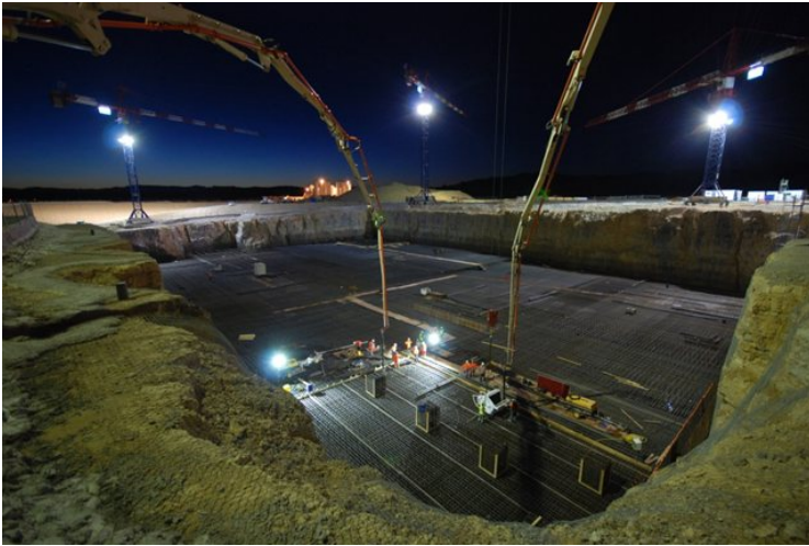
At 5:00 a.m. on Tuesday, 9 August, operations began to create the lower basemat of the Tokamak Complex
