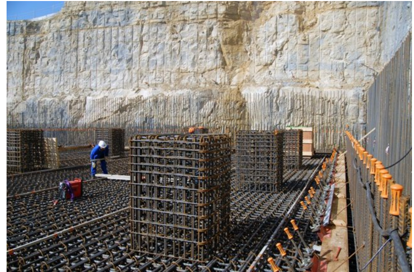
Sitting atop the lower basemat, 500 of these 1.8 metre concrete columns will support the seismic pads. These, in turn, will support the upper basemat of the Tokamak Complex—the actual "floor" of the installation (August 2011).
