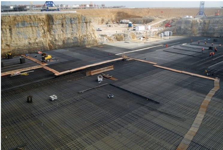
Steel reinforcement bars—each one weighing nearly 100 kilos—are built up to 1.5 meters on the floor of the Seismic Pit. In the distance, the future ITER Headquarters buildings rises above the platform. (August 2011).
