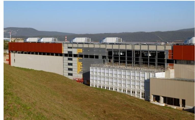
Work advances rapidly on the Poloidal Field Coils Winding Facility in August 2011: the cladding is nearly finished, the three-floor office building is in place.
