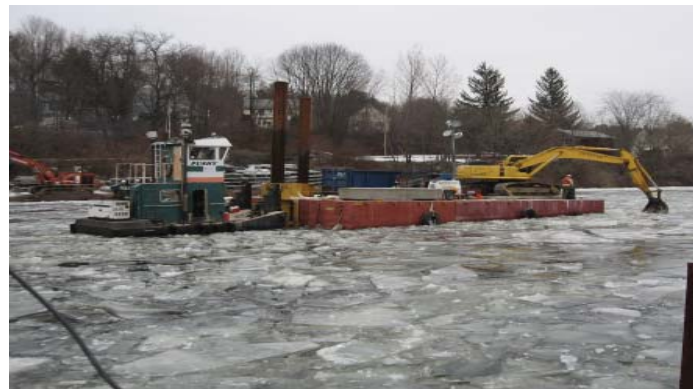
Dredges brave the icy waters of the Cocheco River in April 2007, removing approximately 2,000 cubic yards of rock and 14,000 cubic yards of sediment in the Federal Channel in Dover, N.H.
