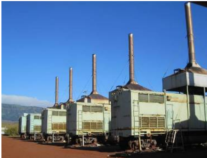
Figure 1-6. 1 MW diesel generators on Lanai, Photo by J. Keller, NREL
