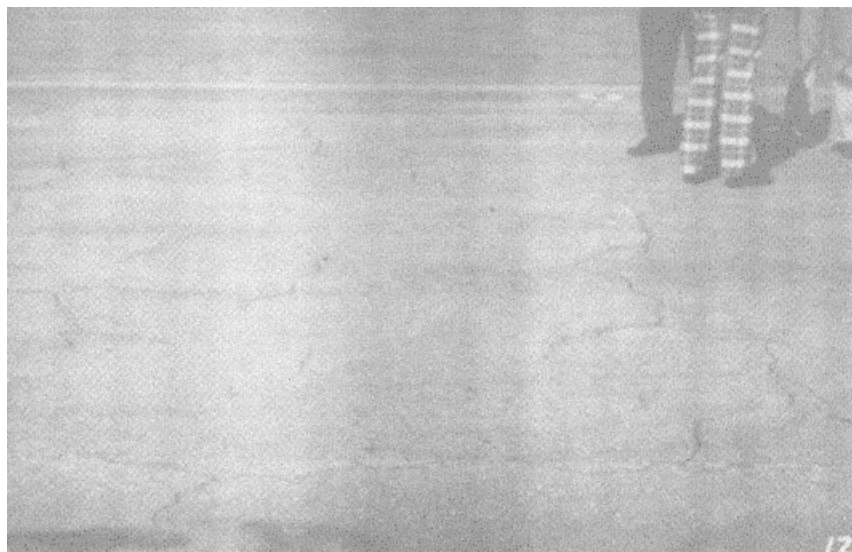
Figure A-10. Low severity block cracking, case 3.
