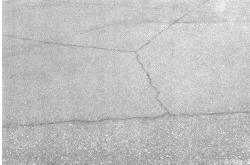
Figure A-23. Low severity joint reflection cracking.
