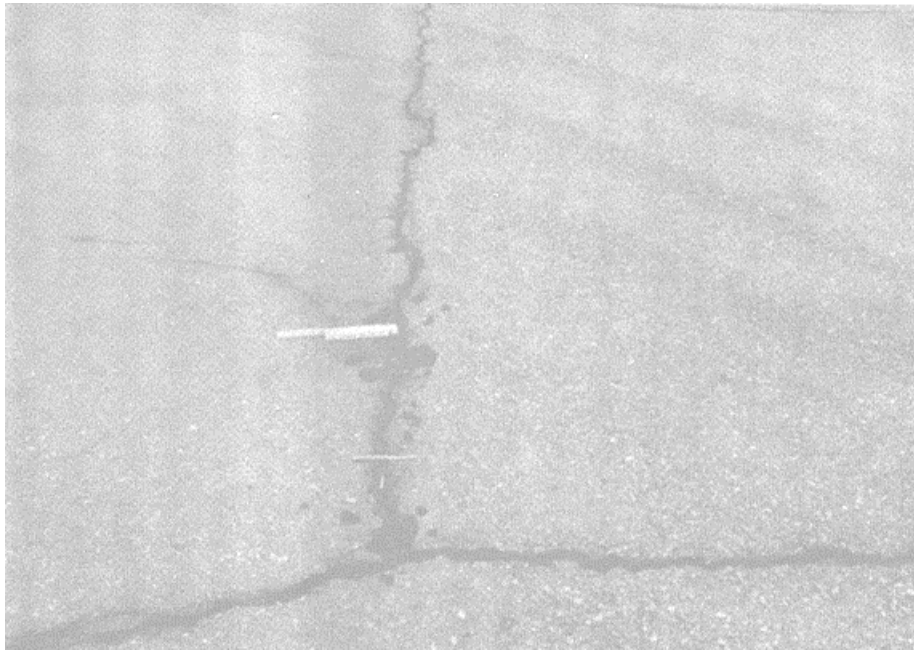
Figure A-24. Medium severity joint reflection cracking case 1.
