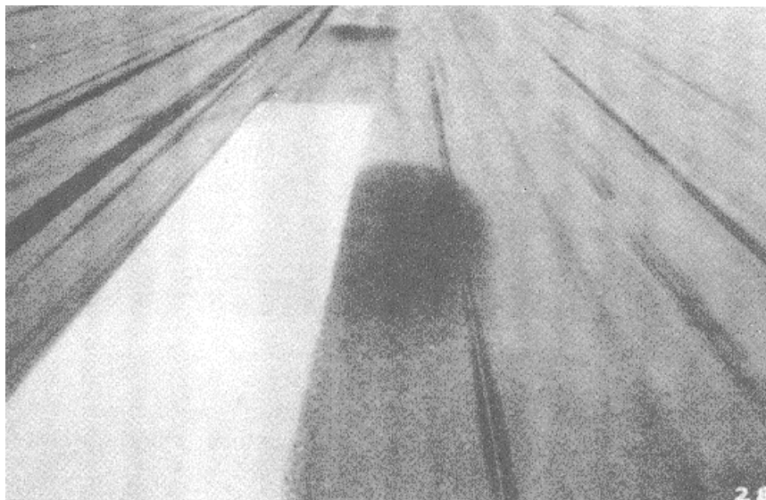
Figure A-21. Jet blast erosion, case 1.
