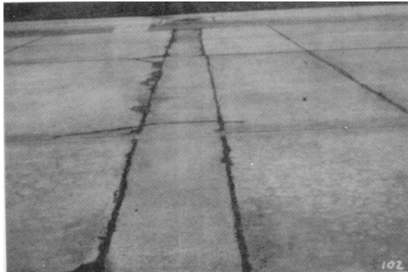
Figure A-98. Low severity utility cut.
