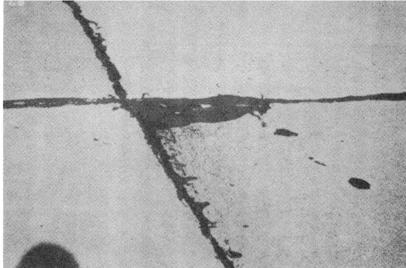
Figure A-83. Low severity D cracking.
