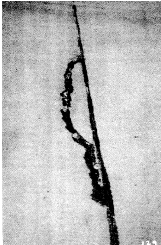
Figure A-125. Low severity Joint spall case 2
