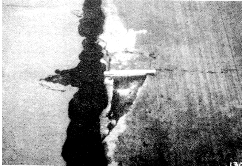
Figure A-126. Medium severity joint spay case 1.
