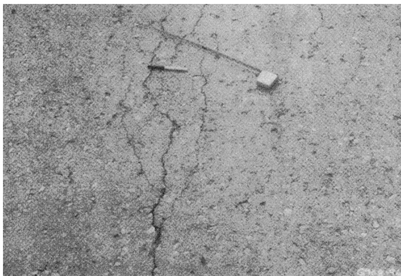
Figure A-1. Low severity alligator cracking, case 1.
