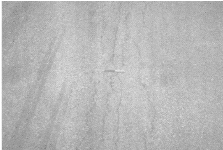
Figure A-3. Low severity alligator cracking, approaching medium severity.
