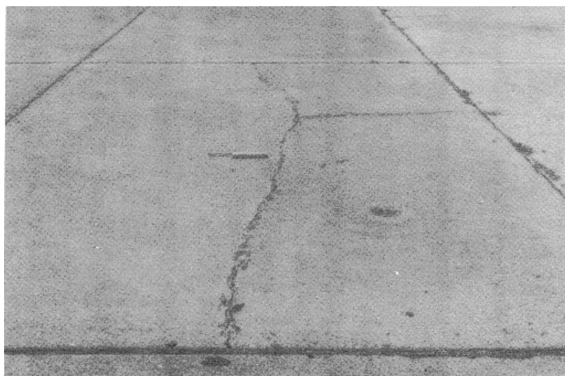
Figure A-82. High severity longitudinal crack, case 2.
