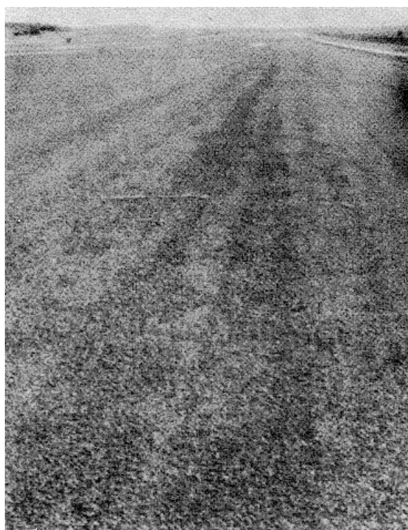
Figure A-49. Medium severity raveling/weathering showing rough and pitted surface in porous friction course pavement.
