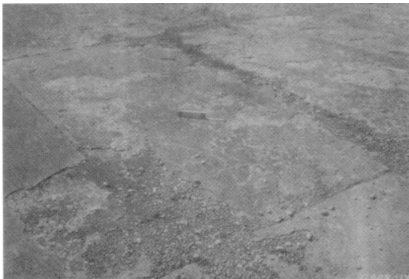
Figure A-109. High severity scaling.
