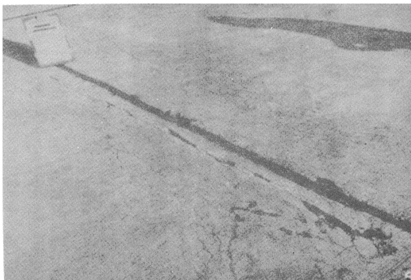
Figure A-86. High severity D cracking.
