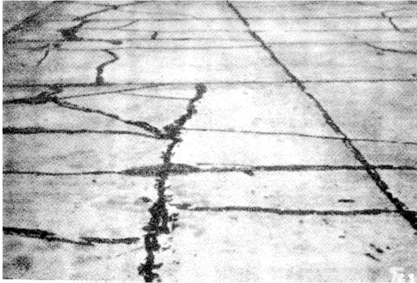
Figure A-121. Shattered slab.
