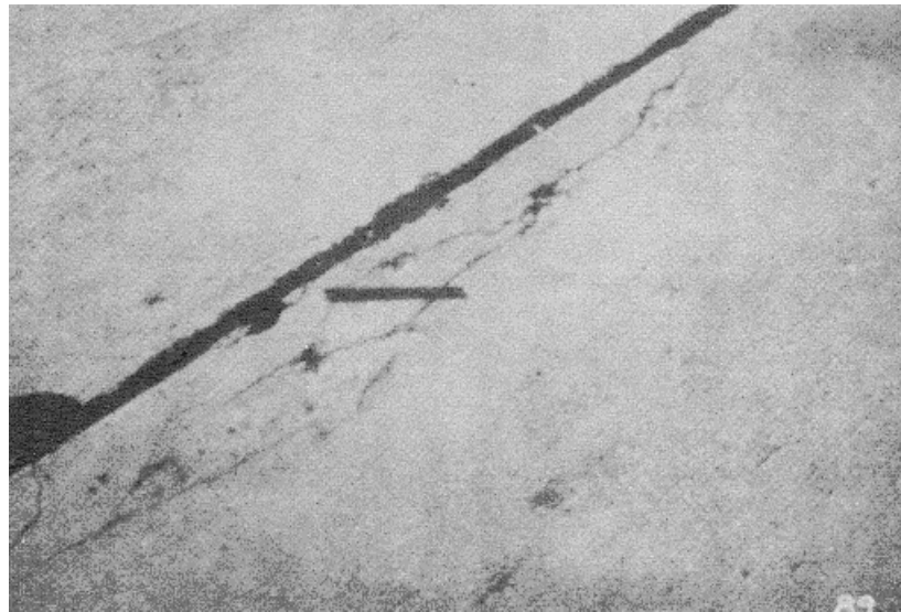
Figure A-85. Medium severity D cracking case 2.
