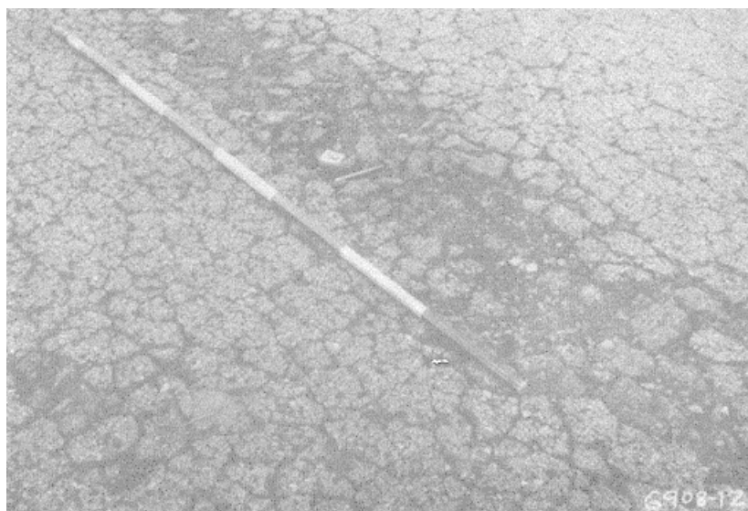
Figure A-6. High severity alligator cracking.
