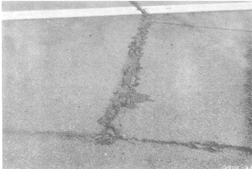
Figure A-26. High severity joint reflection cracking.
