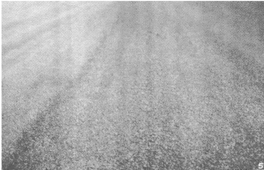
Figure A-43. Low severity raveling/weathering, case 2.
