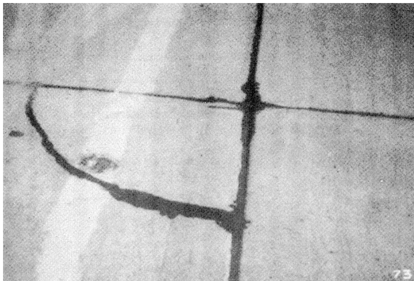
Figure A-69. Low severity corner break, case 1.
