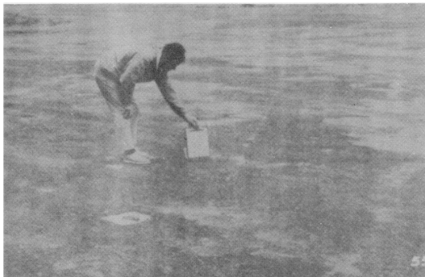
Figure A-50. High severity raveling/weathering.
