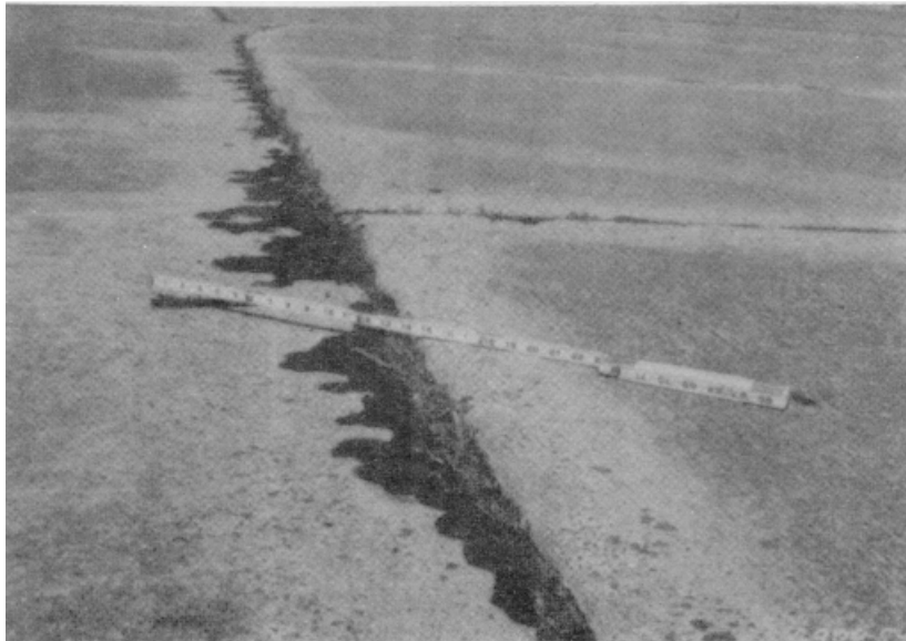
Figure A-113. Medium severity settlement on apron.
