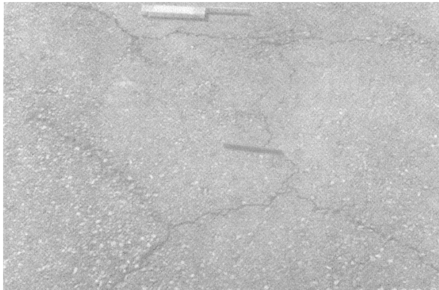
Figure A-9. Low severity block cracking, case 2.
