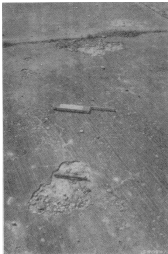
Figure A-110. Close-up of high severity scaling.
