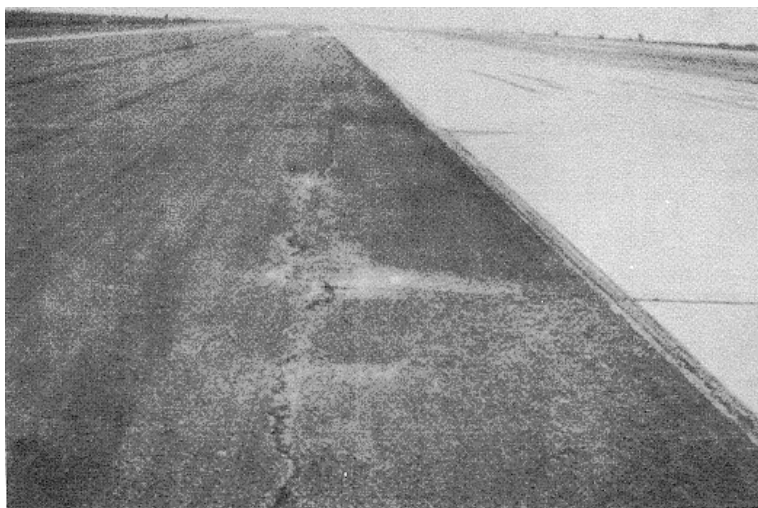
Figure A-58. Low severity shove on the outside and medium severity in the middle.
