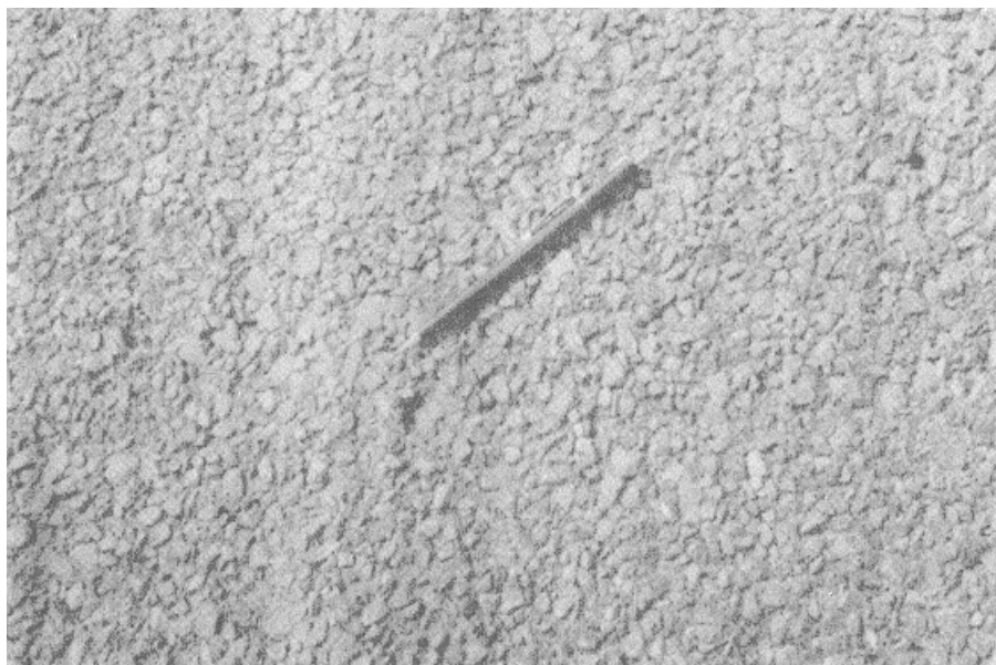
Figure A-46. Low severity raveling/weathering in porous friction course pavement.
