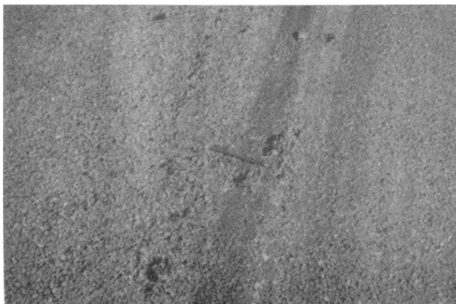
Figure A-51. High severity raveling/weathering in porous friction course pavement.
