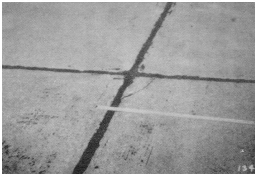
Figure A-130. Low severity corner spall; case 1.
