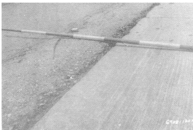
Figure A-59. High severity shoving.
