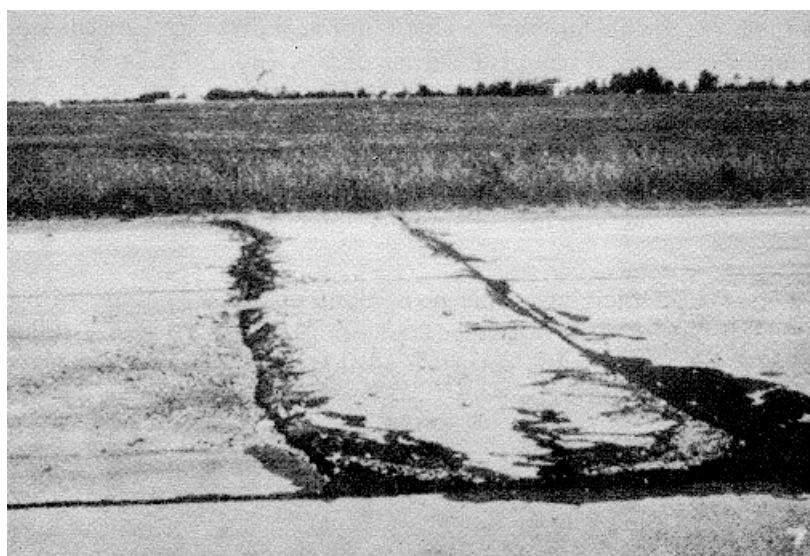
Figure A-67. Medium severity blowup
