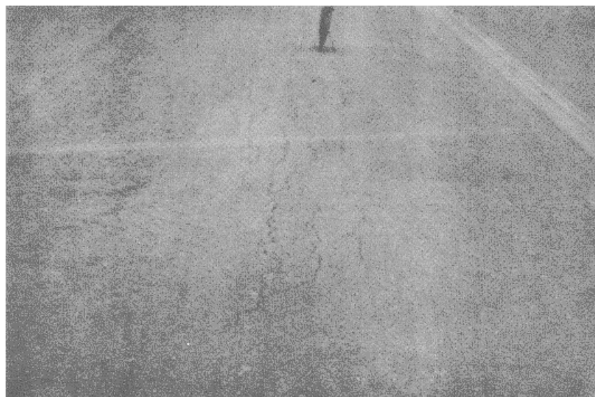
Figure A-2. Low severity alligator cracking, case 2.
