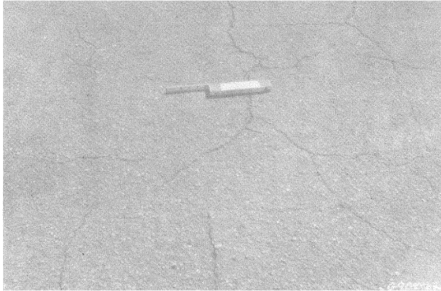
Figure A-8. Low severity block cracking, case 1.
