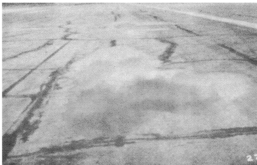
Figure A-20. High severity depression
