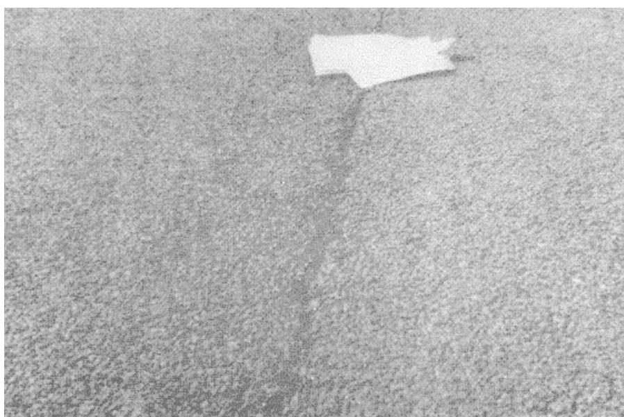
Figure A-34. High severity crack, porous friction course pavement.
