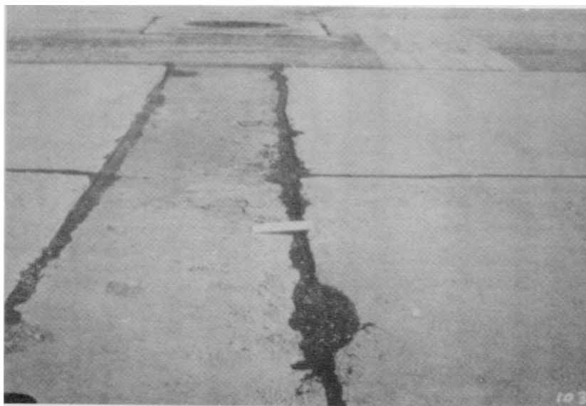
Figure A-99. Medium severity utility cut.
