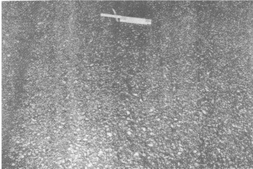
Figure A-42. Low severity raveling/weathering, case 1.
