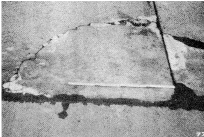
Figure A-73. High severity corner break.
