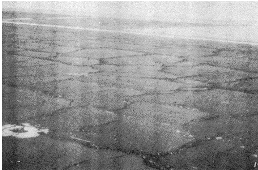
Figure A-14. High severity block cracking case 2.
