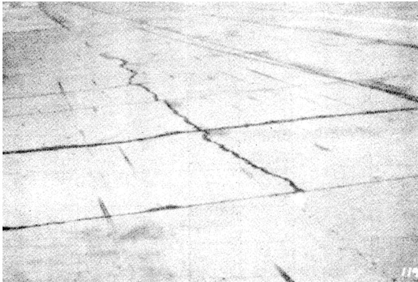
Figure A-120. Medium severity intersecting cracks, case 2.
