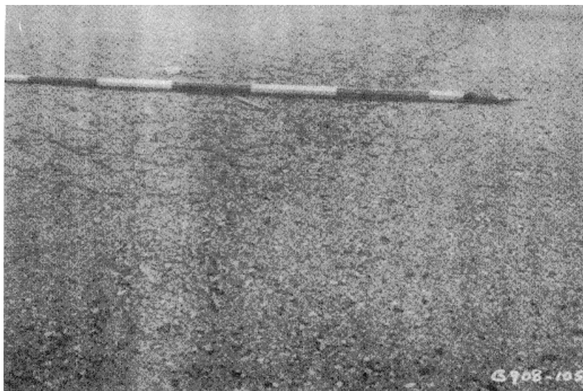
Figure A-17. Low severity depression.
