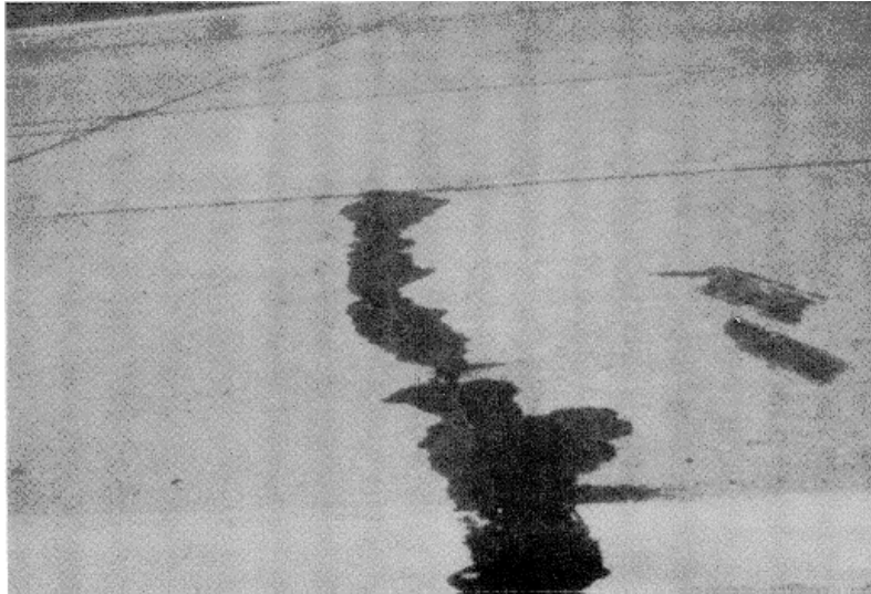
Figure A-79. Medium severity transverse crack, case 2.
