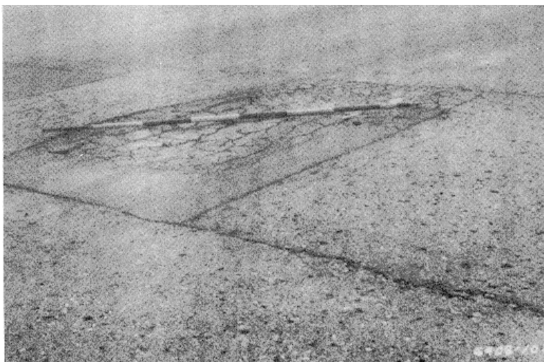
Figure A-40. High severity patch.
