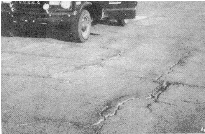
Figure A-13. High severity block cracking case 1.
