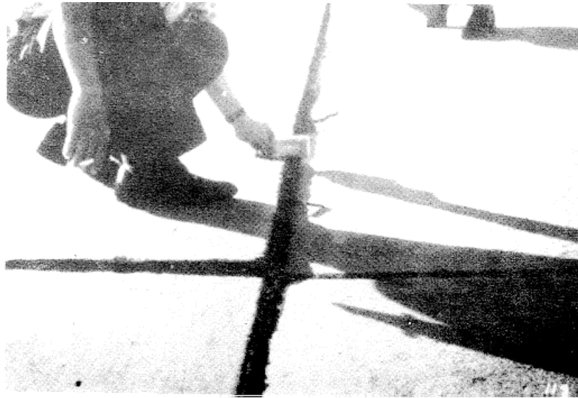
Figure A-115. High severity settlement, case 2
