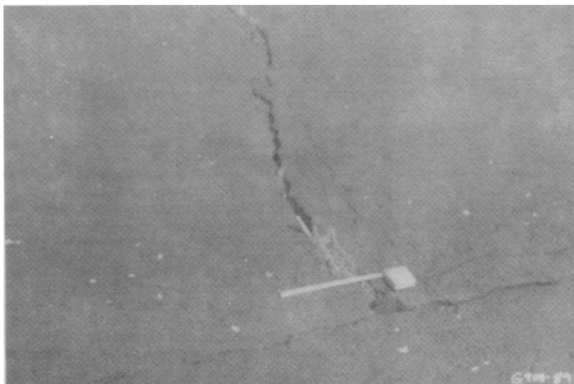
Figure A-33. High severity longitudinal crack.
