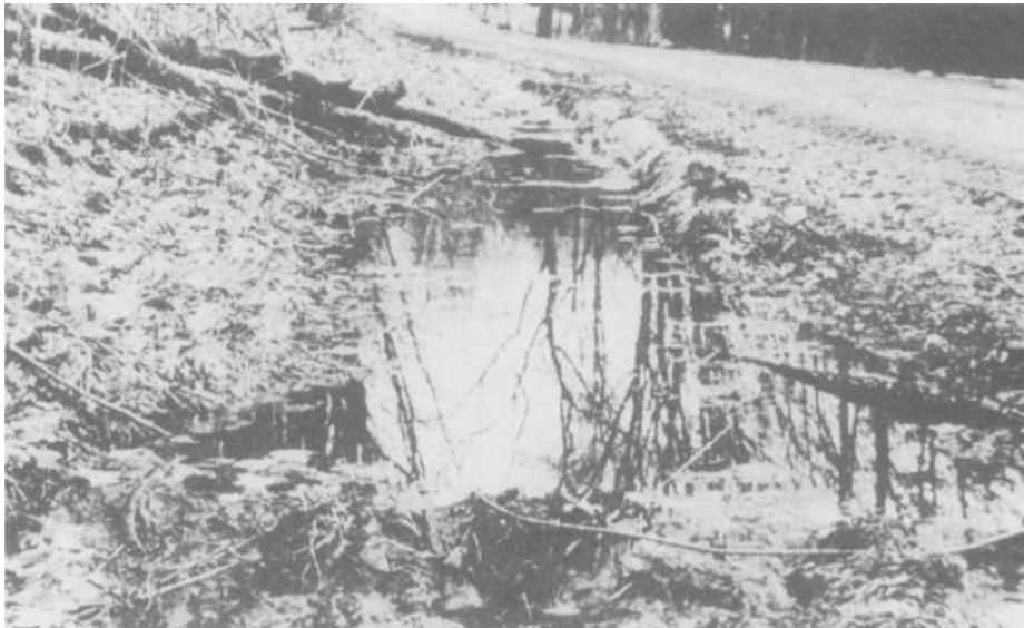
Figure B-4. High severity example of inadequate roadside drainage.
