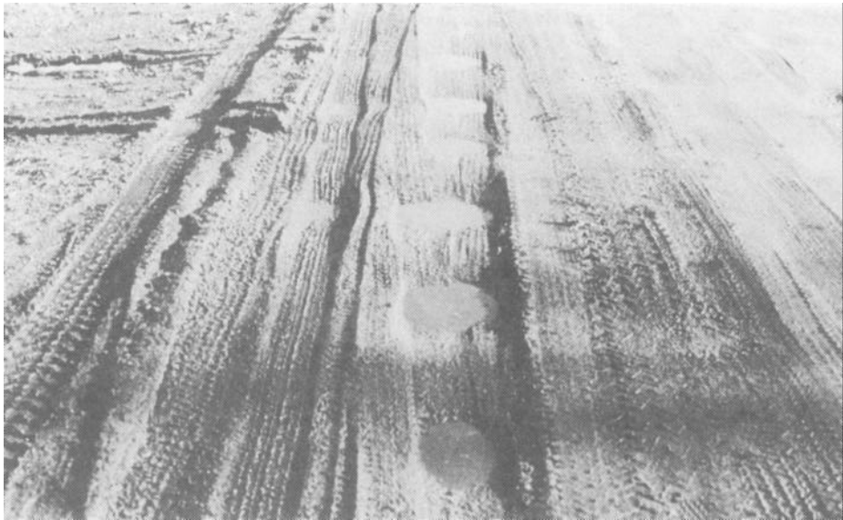
Figure B-6. Medium severity example of corrugations.
