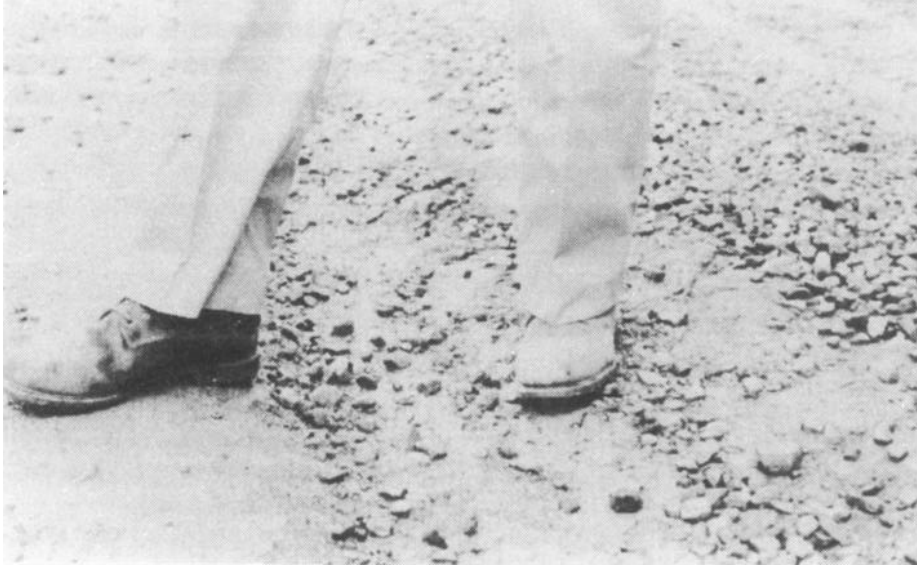
Figure B-14. Low severity example of loose aggregate.
