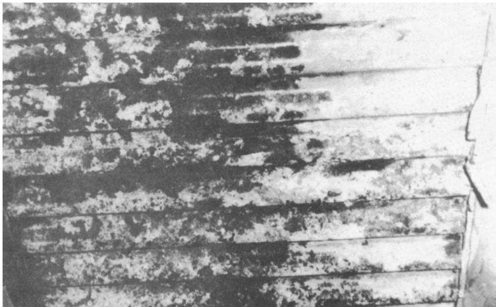
Figure 8-29. Rusted stay-in-place forms underneath a concrete deck.
