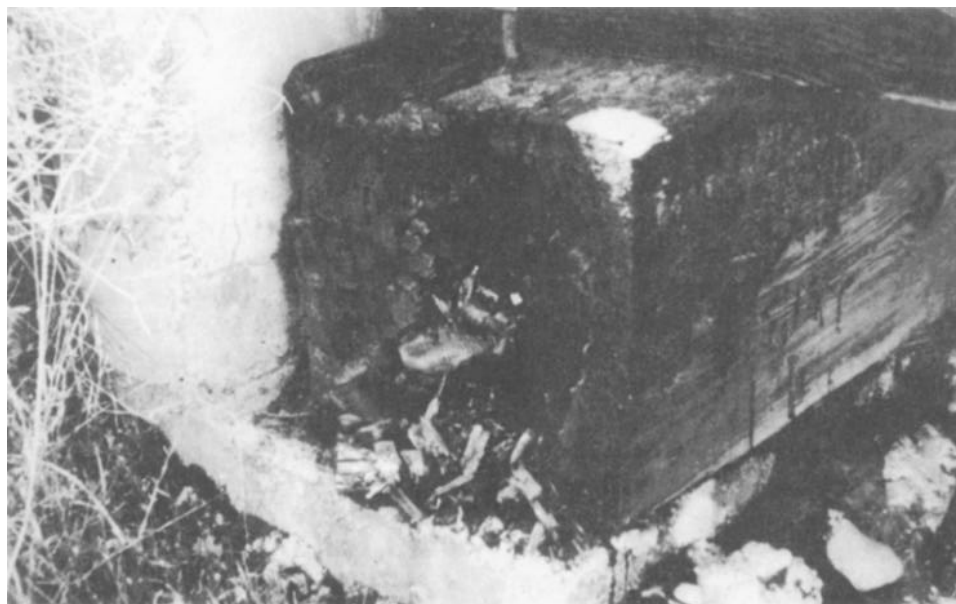
Figure 5-14. Advanced wood decay in crosstie.
