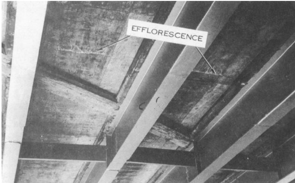
Figure 8-28. Efflorescence on the underside of a concrete deck.
