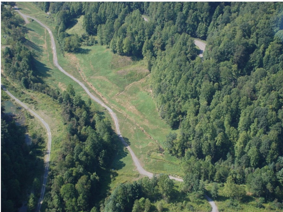
Cranes Nest Gob Pile Removal Project, September 2010. GOBCO, LLC of Abingdon, Virginia completely removed a 9-acre coal waste pile and restored a natural stream channel that had been buried by waste coal. This abandoned mine land project won a national reclamation award from the federal Office of Surface Mining Reclamation and Enforcement.
