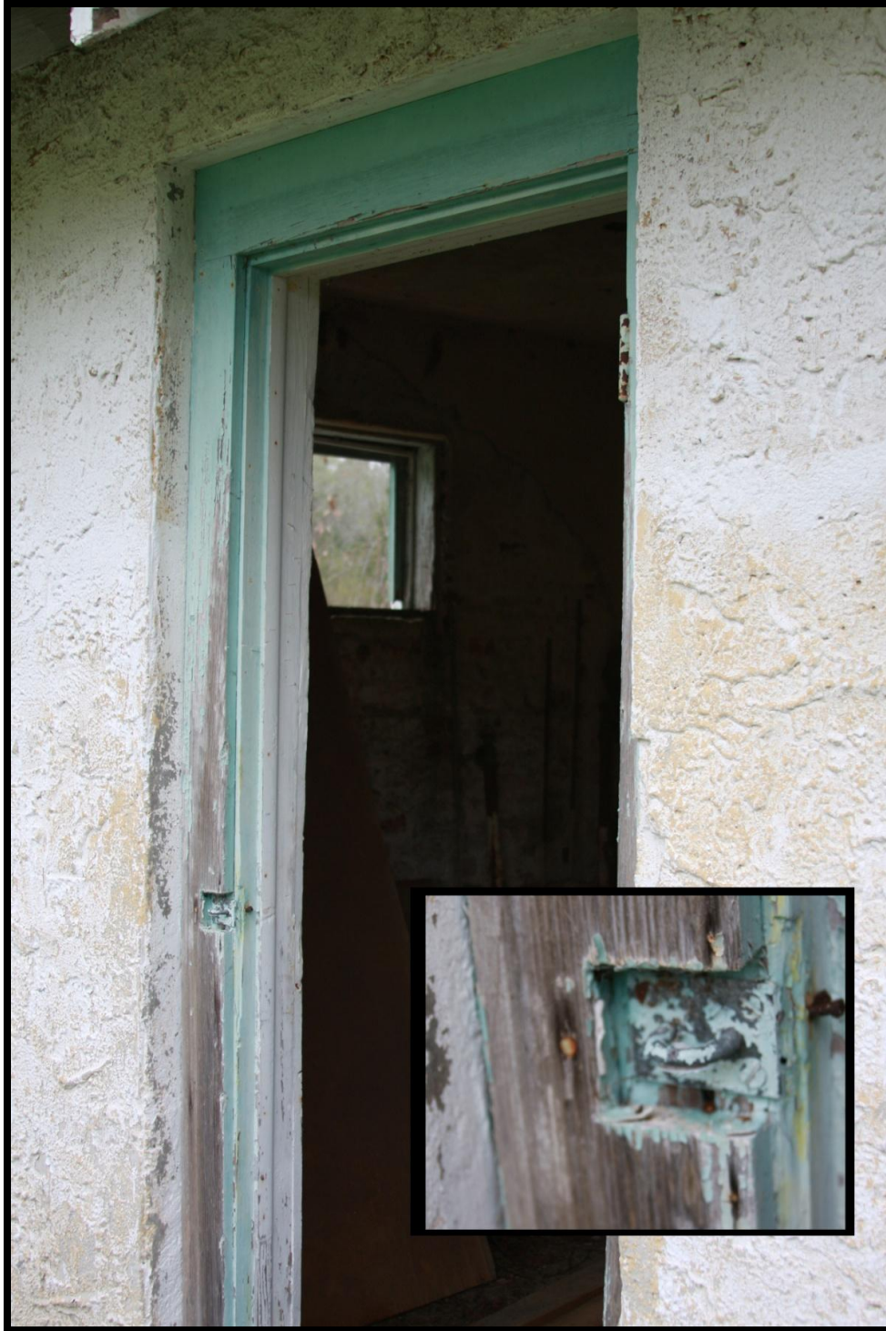
Figure 56. Door frame of confinement cottage showing modification to door when building was converted from storage to confinement cottage and later to the farm manager's office. The door was modified to swing outside, rather than inside. The small window in figure shows former outside latch for lock.
