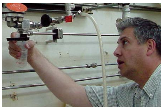
FIGURE 4: Operator Ricky Sprow testing a portion of a newly installed condensate removal system.
