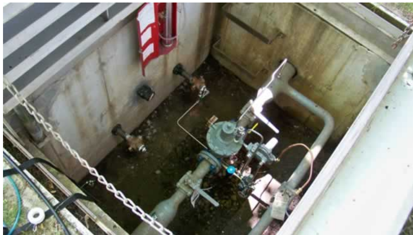
District Regulating Station –Vault Type
