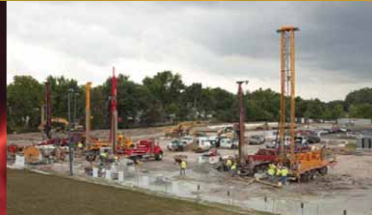
Workers drill boreholes for a geothermal heating and cooling system at Ball State University’s campus in Muncie, Indiana (Photo courtesy of Ball State University)
